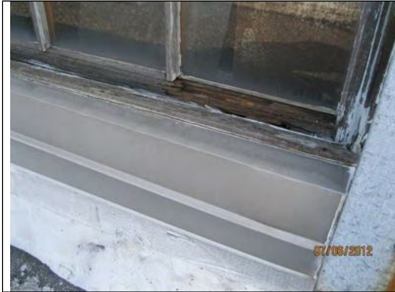
Photo 65: Typical deteriorated wood window frame.
