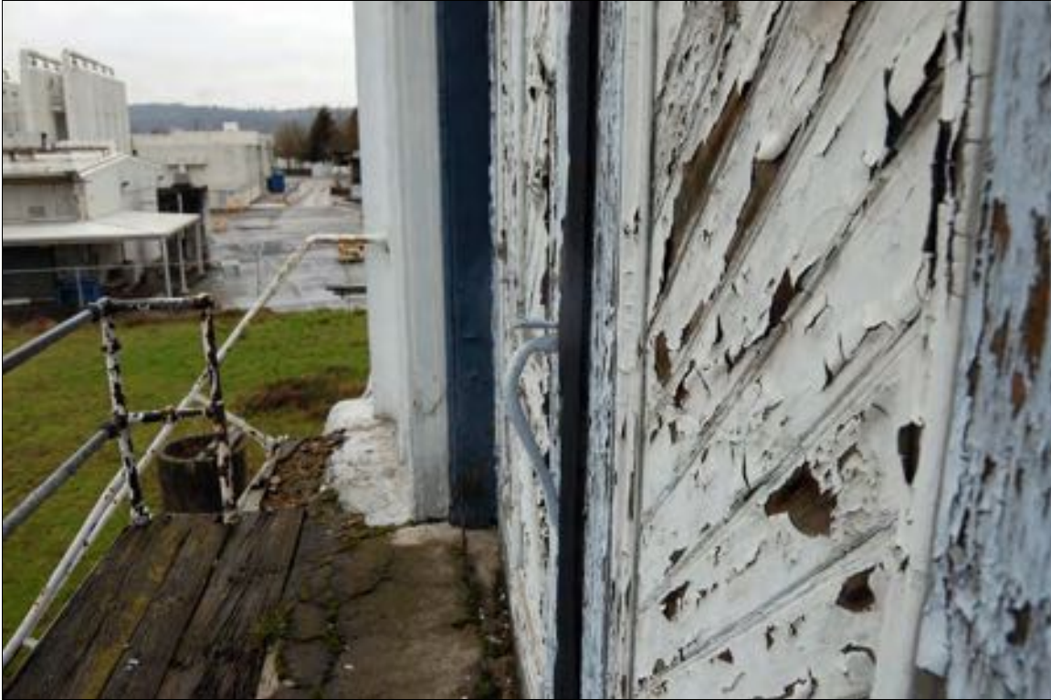
Figure 6. Detail of weathering and deterioration of exterior stair and second level door on southeast side, view to the southwest.
