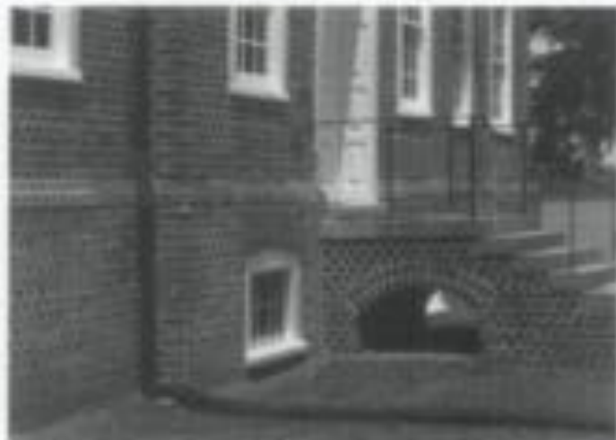
Fig. 17. In testing a theory for the cause of basement wetness, the owner used long black extender pipes to direct roof run-off away from the foundation. This test established that the owner did not need expensive waterproofing of the foundation, but a better drainage system. Photo: David M. Smith.
