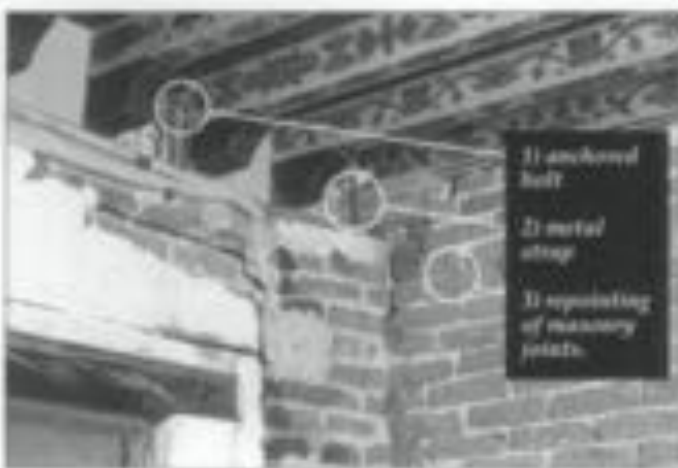
11. Limited intervention should correct obvious structural deficiencies, such as tying vulnerable elements together and repointing masonry. See here in 1) anchored bolt, 2) metal joint strap, and 3) repointing and resurfacing masonry joints. When replastering and painting these reinforcements will not be visible. Photo: Historic Preservation Partners for Earthquake Response.
