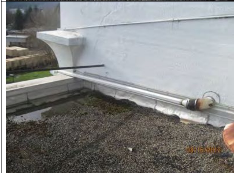
Photograph 22: Drain line penetration from upper roof to low southwest roof is routed over west parapet.
