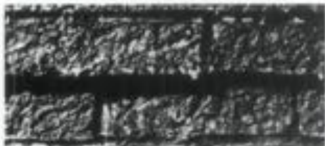
Hazards of Sandblasting and Surface Coating. In order to "protect" this heavily sandblasted brick, a clear surface coating or sealer was applied. Because the air temperature was too cold at the time of application, the sealer failed to dry properly, dripping in places, and giving the brick surface a cloudy appearance.
