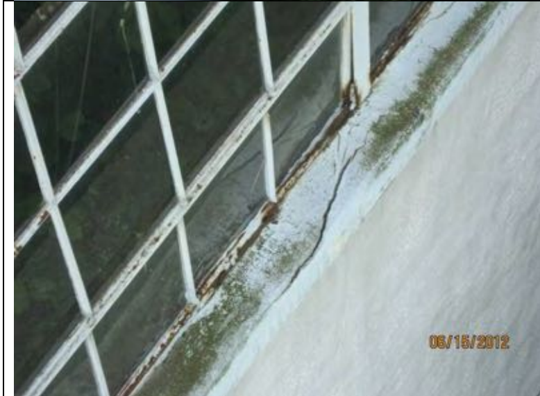
Photo 55: Rusted steel framed window and spalled concrete sill material.
