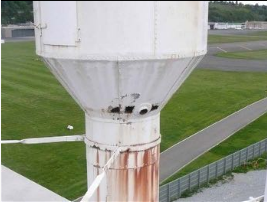
Figure 68: Detail of exhaust vent where the sheet metal has rusted through, providing access for water and pests.
