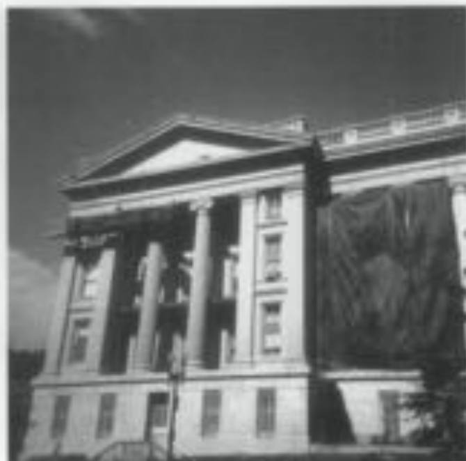
Figure 25. A tarpaulin protects and shields pedestrians from potentially harmful spray while chemical cleaning is underway on the granite exterior of the U.S. Treasury Building, Washington, D.C.
