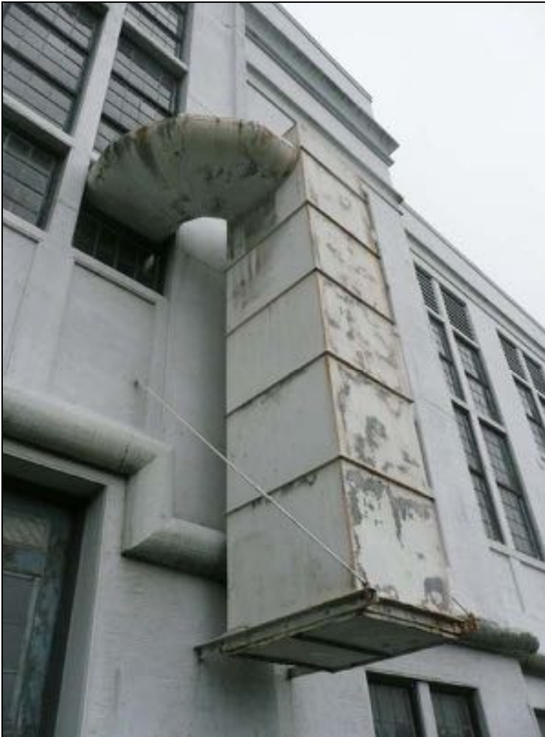
Figure 82: Metal exhaust duct and rusted, deteriorating attachments and support structure on the west side of the Engine Room.
