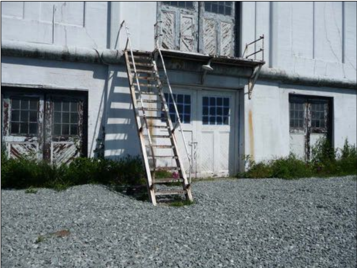
Figure 81: South balcony and stair with deteriorated wood decking and attachments, significant rust, and missing pipe rail elements.
