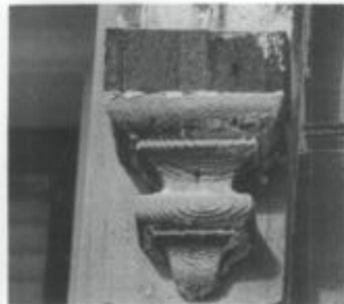
Fig. 12 Sandblasting has permanently damaged this ornamental bracket. Even paint will not be able to hide the deep erosion of the wood. Photo: David W. Look, AIA.
