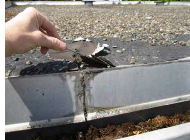
Photo 28: Membrane unadhered at sheet metal lap joint; typical condition.
