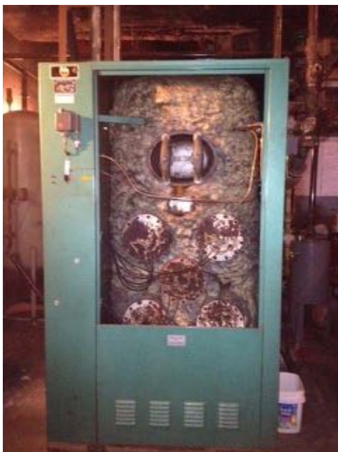
Image 9: Boiler access panel removed
