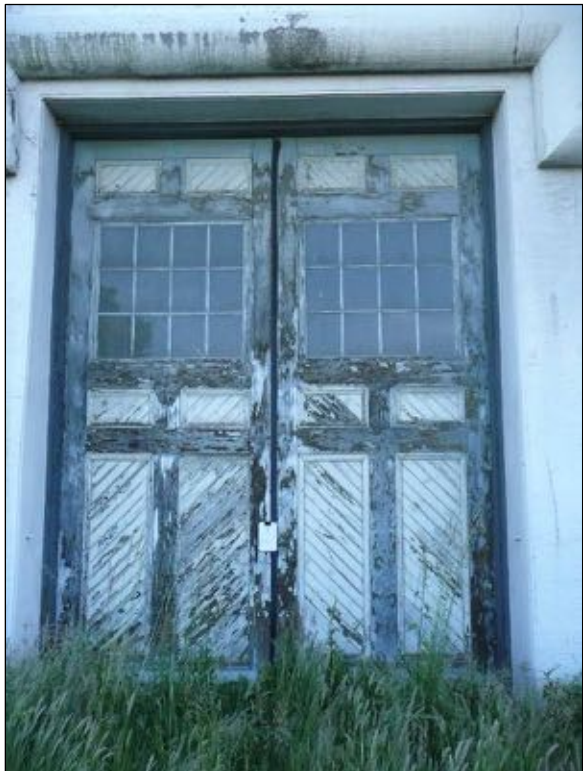
Figure 79: Detail of the large door from the west side of the Engine Room.
