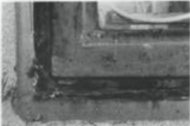
Fig. 6 b. View from the exterior showing the deteriorated condition of the lower corner of a window prior to repair. While the sash was in relatively good condition, the frame behind was rusted to the point of inhibiting operation.
