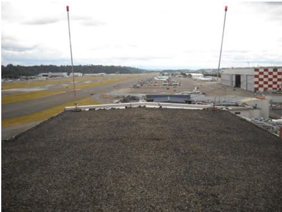
Photograph 10. RF-10: Multi-layer black built-up roofing with pebbles over multi-layered black fibrous material (M)
