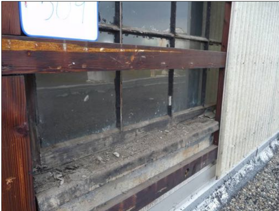
Figure 74: Detail of one of the roof monitor windows, on the south side, showing evidence of previous repairs and waterproofing attempts, including parging over the wood frame, and mastic applied over the frame and glass.
