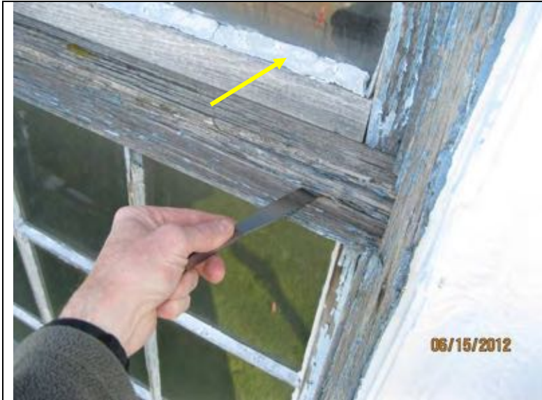
Photo 37: Wood window frames are deteriorated to varying degrees, worst at west and south elevations. Note glazing putty holding the glazing in place where the arrow points.
