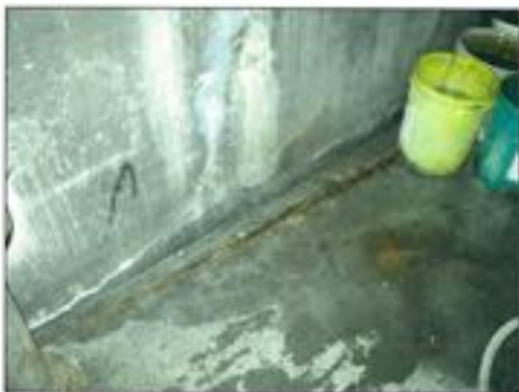
Figure 1-8: Top slab reinforcement corrosion at the second floor on the west street bay.
