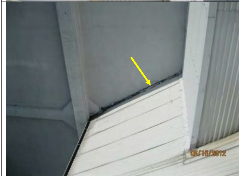
Photo 34: Lower corrugated metal roof with roofing material butting to concrete wall. Mastic has been applied at the joint.
