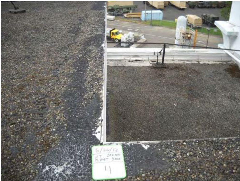
Photograph 4. RF-4: Black roll-down roofing over silver foil over black asphaltic sealant over multi-layered black felt (M)
