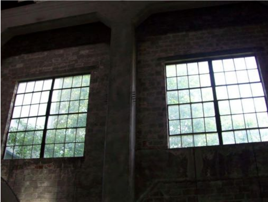
Photograph 17. HSA 13: Window putty glazing (M)
