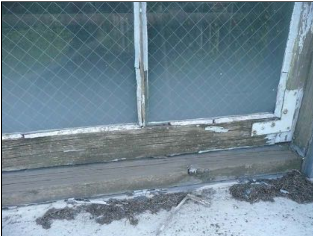
Figure 72: Detail of the sill of a ground floor window, with open grain, checked sill, and loose joint at the stile/bottom rail.
