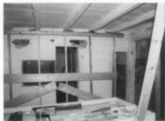
Figure 6. Interior bracing which will last the duration of the mothballing will protect weakened structural members. Jellie Coffin House. Photo: John Miller Architects.
