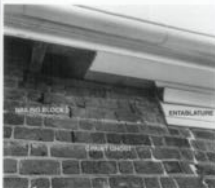
Figure A. Careful examination of the masonry reveals different periods of construction and repair through the composition and detailing of bricks and mortar. Depending upon location, open vertical joints may indicate the location of walling blocks for decorative trim or weeps for drainage. These open joints at the building's cornice show evidence of an earlier window rehabilitation extending down two courses below the present trim. The paint ghosts below the lowest bricks confirm the entablature's existence and provides clues to its size and finish.
