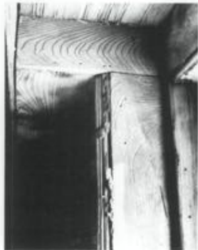
Abrasive Cleaning of Wood. This wooden window sill, molding and paneling have been sandblasted to remove layers of paint in the rehabilitation of this commercial building. Not only is some paint still embedded in cracks and crevices of the woodwork, but more importantly, grit blasting has actually eroded the summer wood, in effect raising the grain, and resulting in a rough surface.
