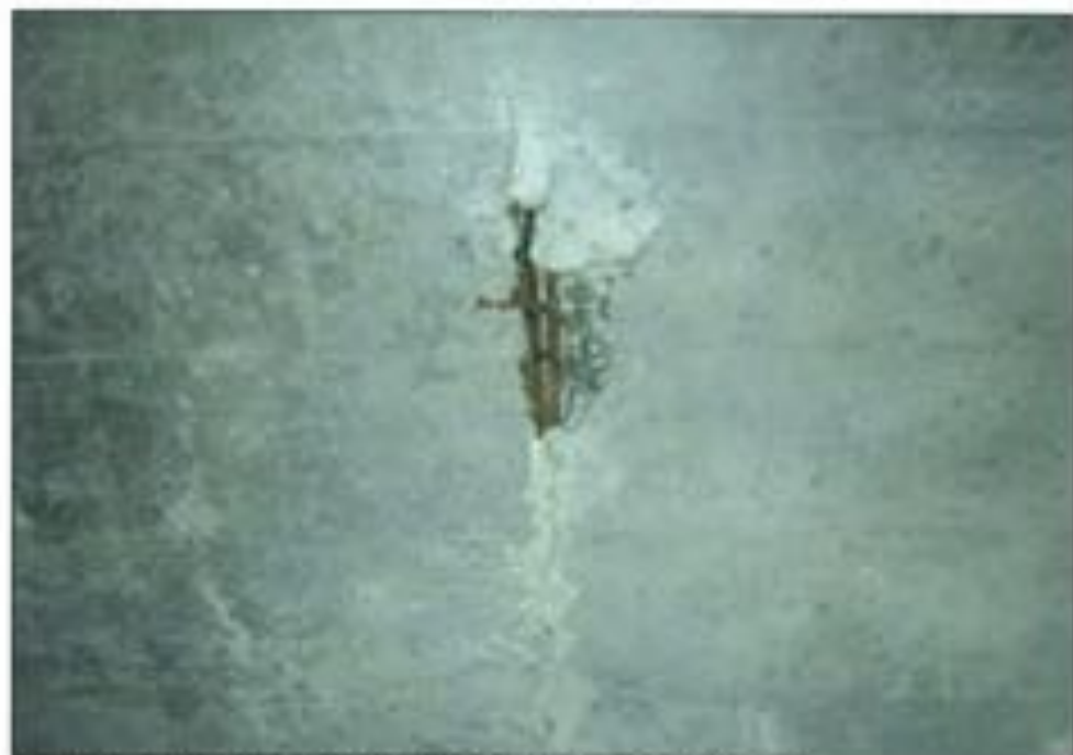
Figure 1-7: Concrete spalling and corrosion of embedded conduit or reinforcement.
