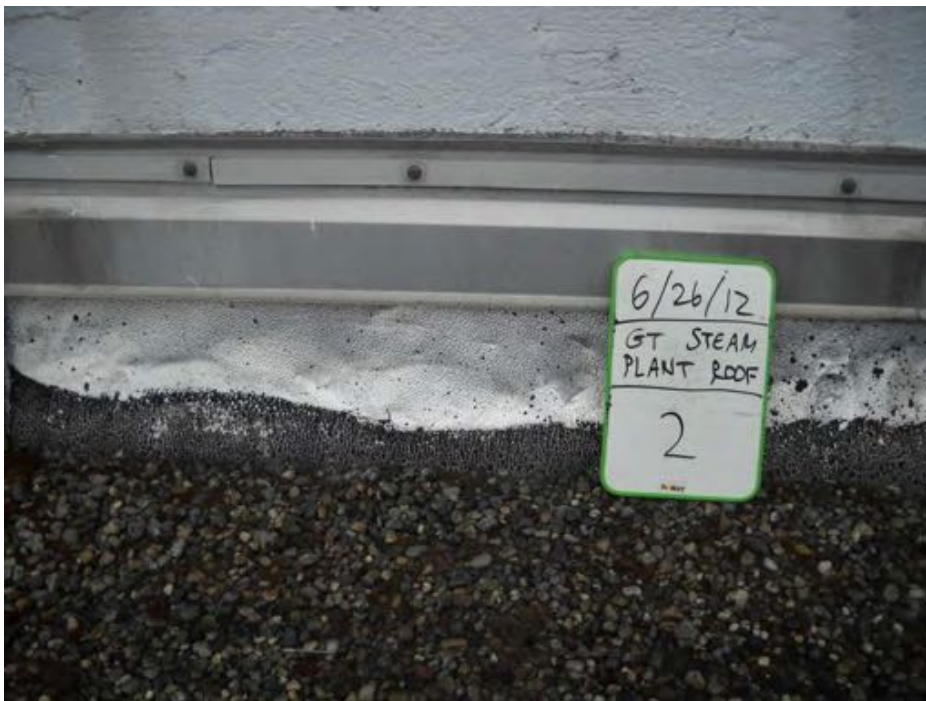
Photograph 2. RF-2: Black roll-down roofing over silver foil over black asphaltic sealant over multi-layered black felt (M)
