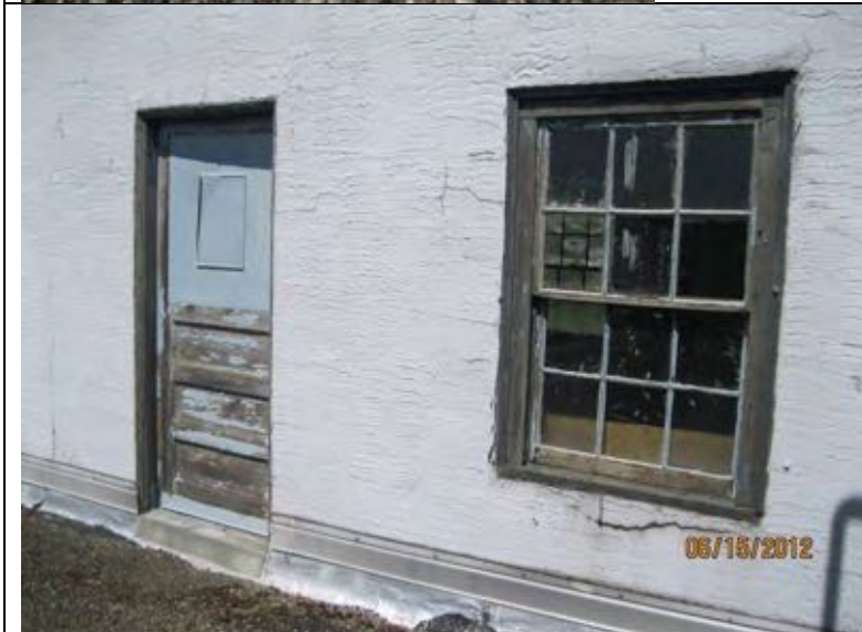
Photograph 7: East end of NW roof with access door. Note parge coat over hollow clay tile is cracked and spalling around the window.
