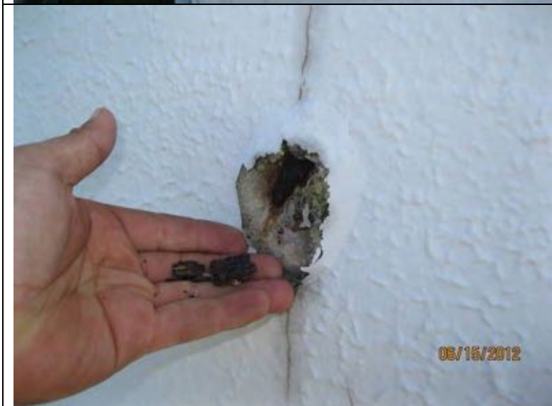
Photo 38: Spalled concrete on west wall, towards the south end, with rusted reinforcing steel in hand.
