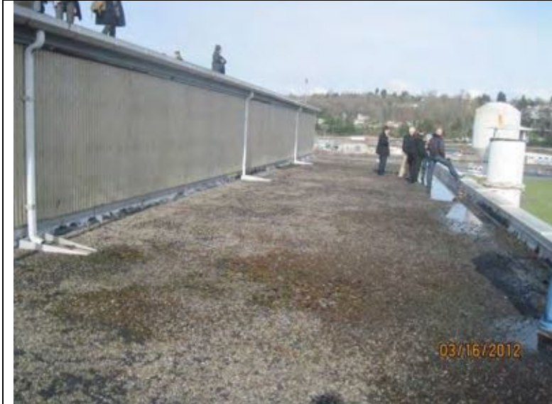
Photograph 15: Overview of roof to the south of the upper north roof, looking east.
