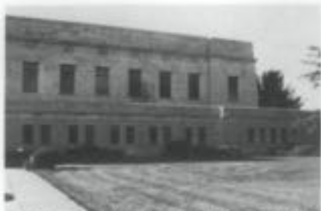
Fig. 6 a. View of the flanking wing of the State Capitol where the rolled steel casement windows are being removed for repair.
