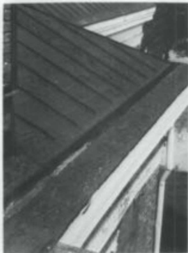
Repeated repair with asphalt, which cracks as it hardens, has created a herringbone surface on this sheet metal roof and built-in gutter, which will retain water. Repairs could be made by carefully heating and scraping the surface clean, repairing the holes in the metal with a flexible mastic compound or a metal patch, and coating the surface with a fiber paint. (Hwane County Courthouse, Kingsport, Tennessee, photo courtesy of Building Conservation Technology, Inc.)
