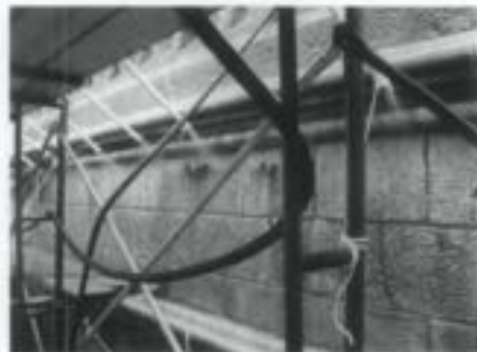
Figure 6. Timed water soaking can be very effective for cleaning limestone and marble as shown here at the Marble Collegiate Church in New York City. In this case, a twelve-hour water soak using a multi-nozzle manifold was followed by a final water rinse. Photo: Hans T. Eason, Wm. Jannoy, Ebers Associates, Inc., N.Y., N.Y.
