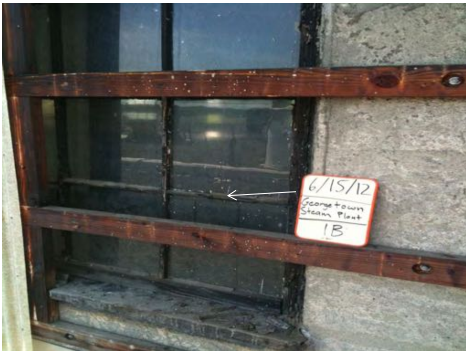
Photograph 4. HSA 1B: Black asphaltic patching material and beige window putty glazing (M)
