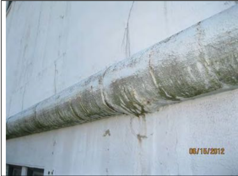
Photo 39: ½ round cornice at west elevation with cracks and spalls at underside.
