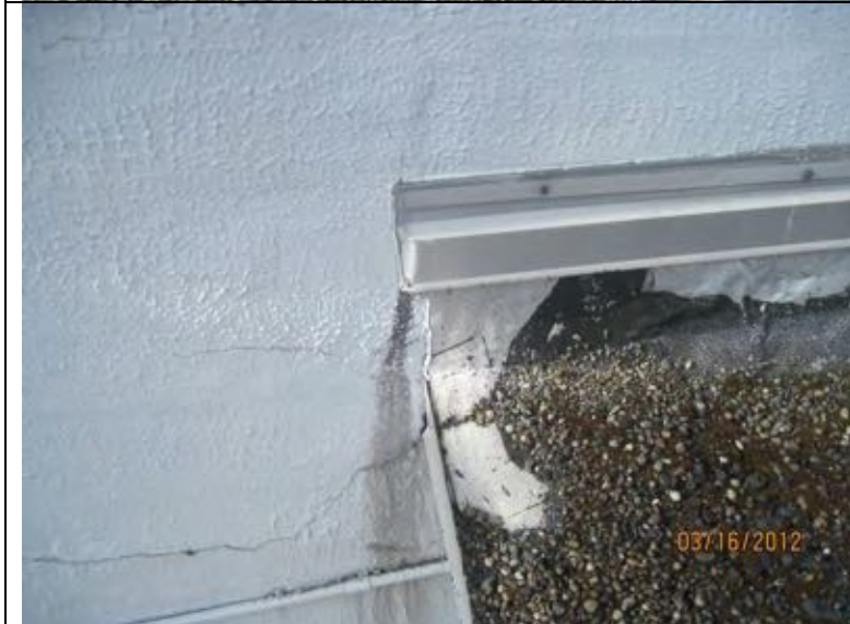
Photograph 24: Typical transition where embedded edge metal meets rising wall is improperly detailed. There needs to be a soldered flashing to receive the cant strip and the counterflashing needs to extend beyond the edge of the roof.
