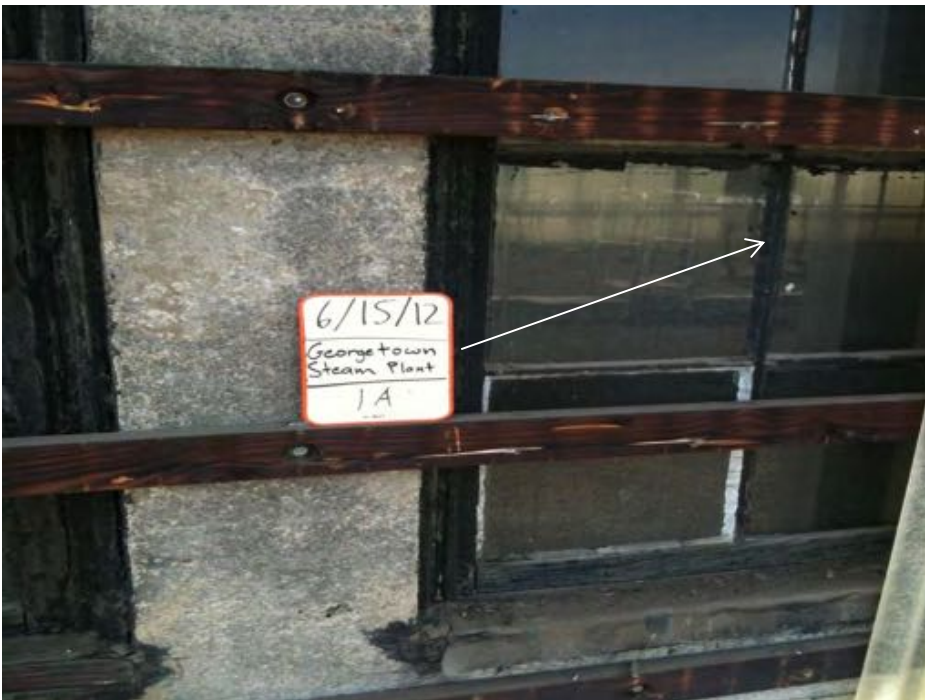
Photograph 2. HSA 1A: Grey/tan window putty glazing with black asphaltic patching material (M)
