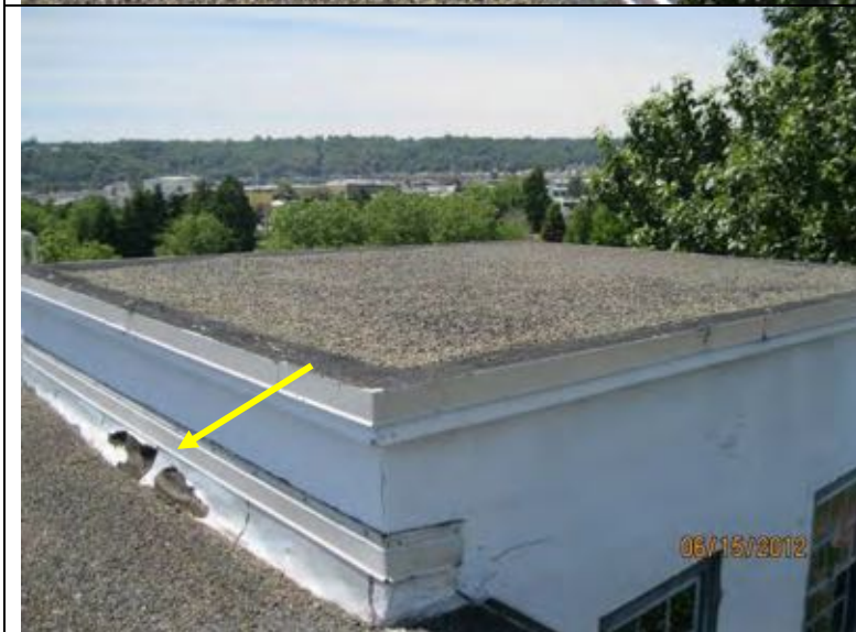
Photograph 10: Note foil facing peeling from baseflashing and blister in baseflashing at same location (arrow).
