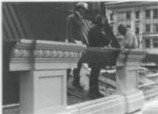
Illus. 18. Substitute materials must be properly installed to allow for expansion, contraction, and structural security. The new balustrade (a polymer concrete modified with glass fibers) at Carnegie Hall, New York City, was installed with steel structural supports to allow window-washing equipment to be suspended securely. In addition, the formulation of this predominantly epoxy material allowed for the natural expansion and contraction within the pre-designed joints. Photo: Courtesy of MIM Studios.
