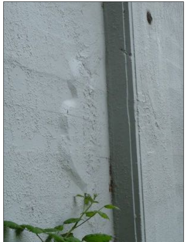
Figure 52: Detail from the east wall, showing a previous patch that has delaminated again. Also visible is the typical incised corner detail.
