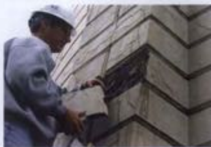
Figure 14. Layers of architectural concrete that have debonded (spalled) from the surface were removed from a historic water tank during the investigation performed to assess existing conditions. Photos: Anita Washko, WSP, January, EITner Associates, Inc.
