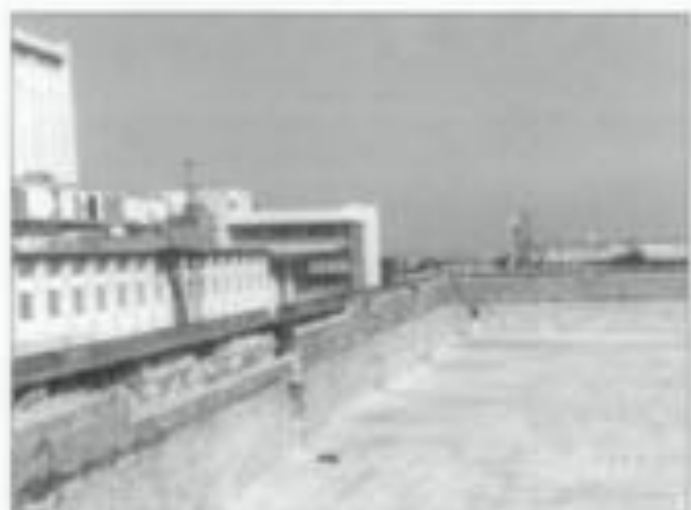
15. The use of fiber composite materials can enhance the shear capacity of existing structural components—beams, columns, and surface elements, such as walls and floors. In this roofing application, the existing roof diaphragm is being strengthened and there is additional benefit to the shear reinforcement of the parapet wall. Photo: The Crosby Group.
