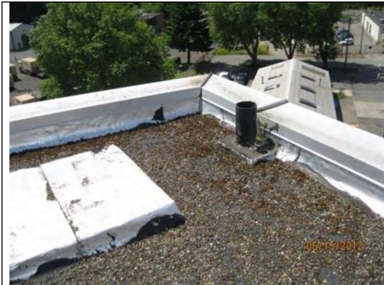
Photograph 3: NW roof with two pipe penetrations in a pitch pocket at the corner. Pitch pockets should not be utilized if possible as they require maintenance.
