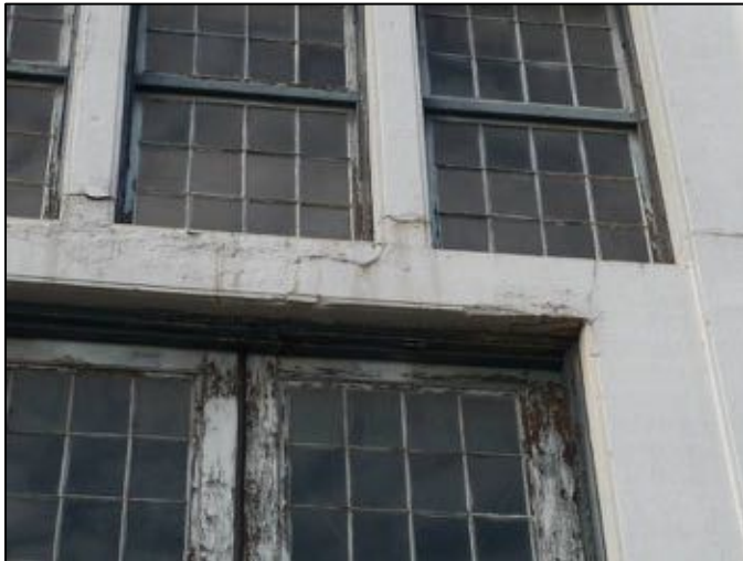
Figure 47: Example of coating cracks, concrete spalls and wood window deterioration.
