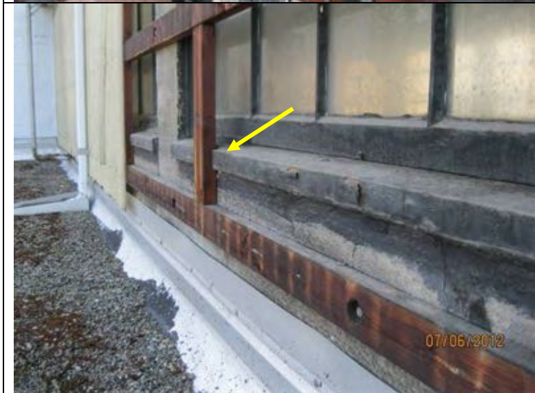
Photo 64: Notched windowsill at clerestory windows for wood framing fit.
