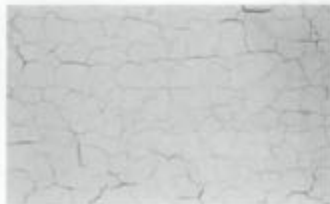
Fig. 5 Cracking—or surface cracking—is an exterior surface condition which can be successfully treated by sanding and painting. Photo: Courtesy, National Decorating Products Association.
