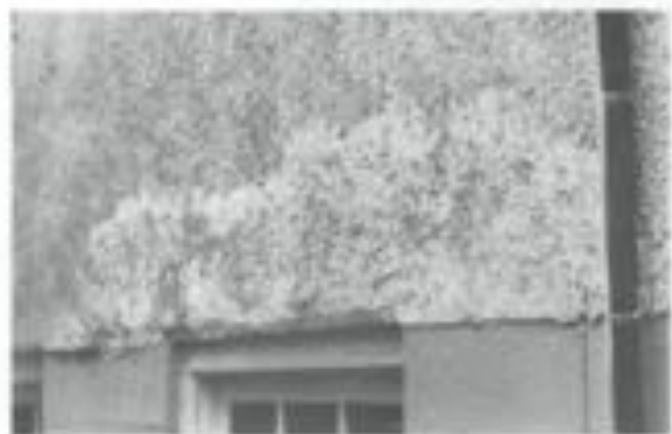
Fig. 14. This poorly executed patch is not the work of a professional plasterer. While it may serve to keep out water, it does not match the original surface, and is not an appropriate repair for historic stucco. Photo: Bethy Christensen.
