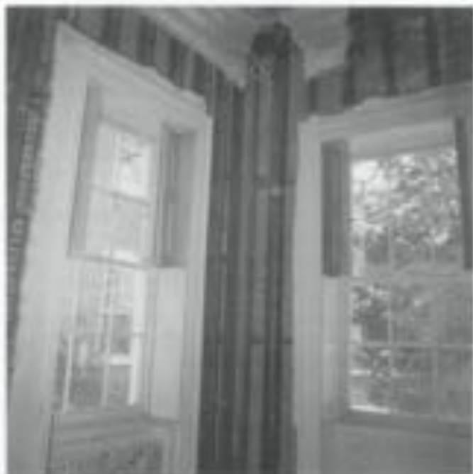
5. The installation of vapor barriers in walls of historic buildings is an effort to control interior moisture and can cause serious damage to historic finishes as shown here. In this example, all the wall plaster and lath have been stripped in preparation for a vapor barrier prior to replastering. Controlling interior temperature and relative humidity can be more effective than adding insulation and vapor barriers to historic perimeter walls. Photo: David A. Conrad, P.E.
