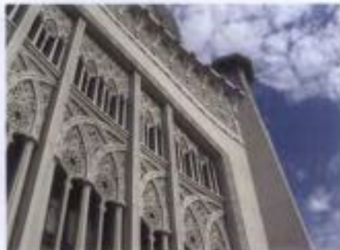
Figure 4. The highly ornamental concrete panels on the exterior facade of the Baha'i House of Worship in Wilmette, Illinois, illustrate the work of fabricator John J. Larley, known as "the man who made concrete beautiful."
