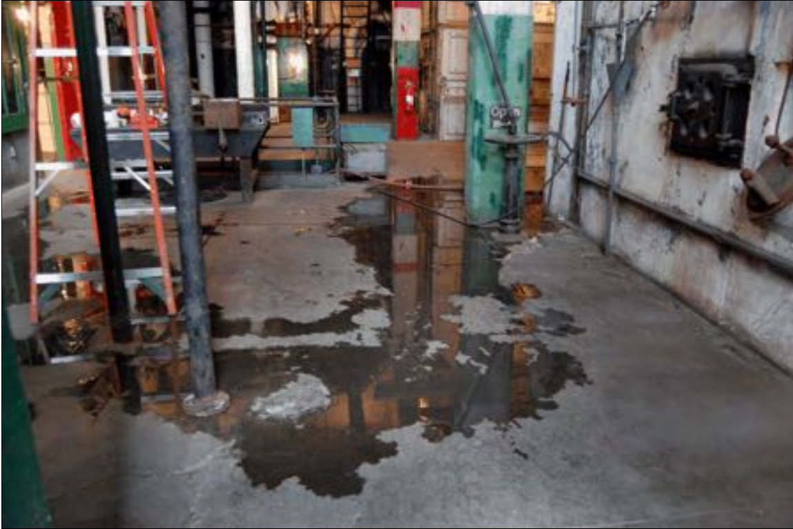
Figure 4. Water pooling at northwest end of boiler room due to roof drain leaks.
