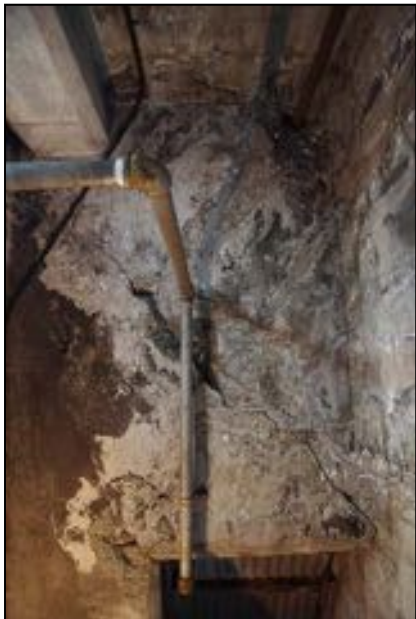
Figure 1-1: Possible Delaminated Concrete Slab Soffit over Stair
