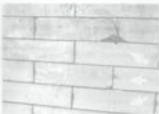
Figure 11. Rinsing with high-pressure water following chemical cleaning has left a horizontal line of abrasion across the bricks on this late-19th century row house.
