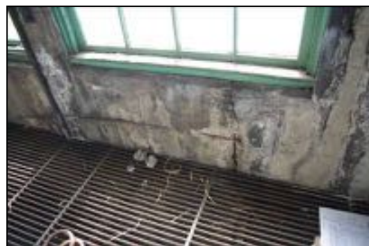
Figure 1-5: Concrete Deterioration below Window Sill
