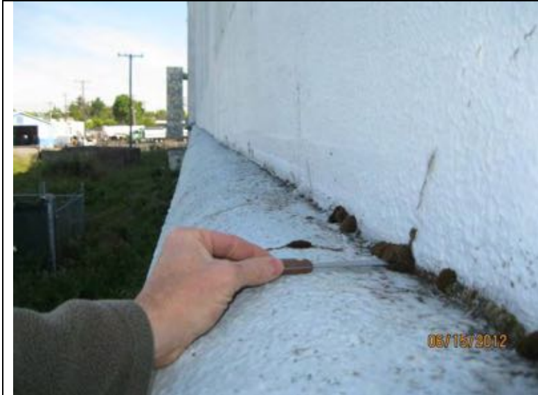
Photo 40: Moss growth at top of ½ round cornice. It appears the top holds moisture.
