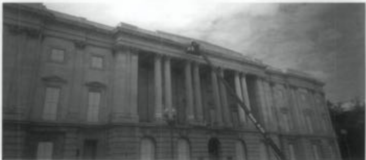
Figure 1. Low-pressure steam (hot pressurized water washing), is being used to clean the exterior of the U.S. Tariff Commission Building, the first marble building constructed in Washington, D.C., in 1838. This method was selected by an architectural conservator as the "gentlest means possible" to clean the marble. Steam can soften heavy scaling deposits such as those on the cornice and column capitals, and facilitate easy removal. Note how these deposits have been removed from the right side of the cornice which has already been cleaned.
