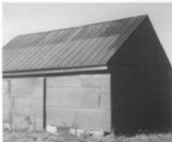
Figure 9. Severely deteriorated wooden siding on a farm building has been covered over with painted plywood panels as a temporary measure to eliminate moisture penetration to the interior. Foundation vents and floor floor boards allow air to circulate inside.
