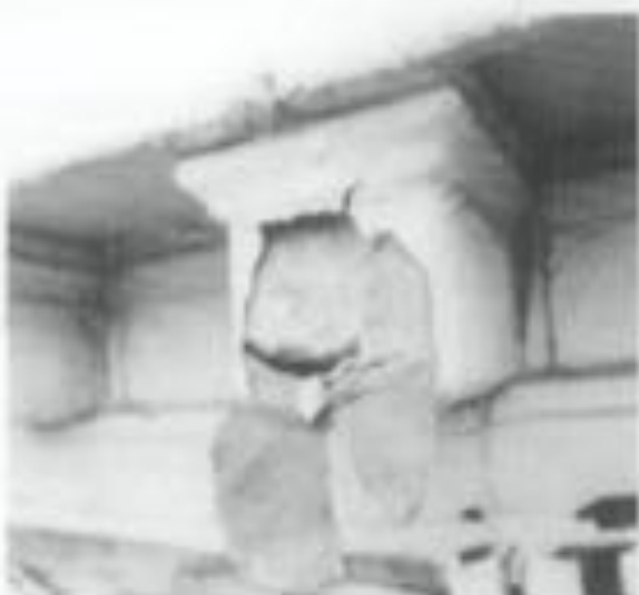
Figure 27. Instead of correcting the roof drainage problems, an elastomeric coating was applied to the already saturated limestone cornice. An elastomeric coating holds moisture in the masonry because it does not "breathe" and does not allow liquid moisture to escape. If the water pressure builds up sufficiently it can cause the coating to break and pop off as shown in this example, often pulling pieces of the masonry with it. Photo: National Park Service Files.
