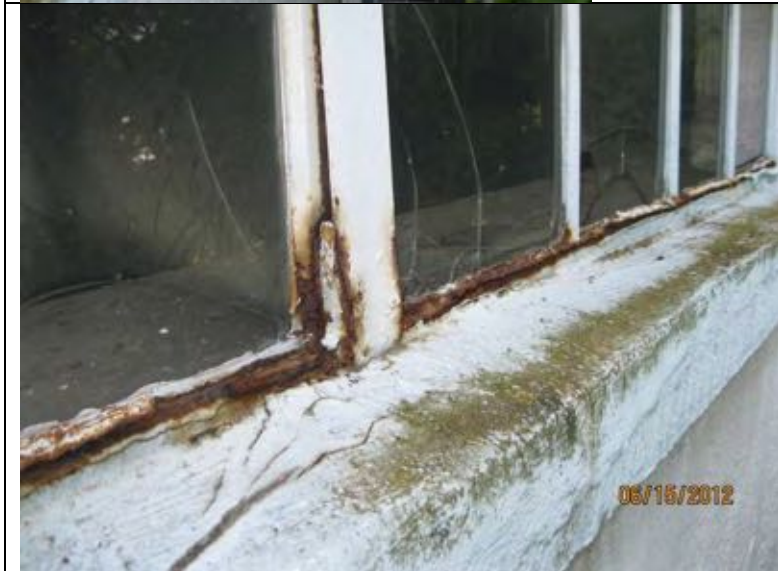
Photo 57: Rusted steel window at north elevation of 1918 addition.
