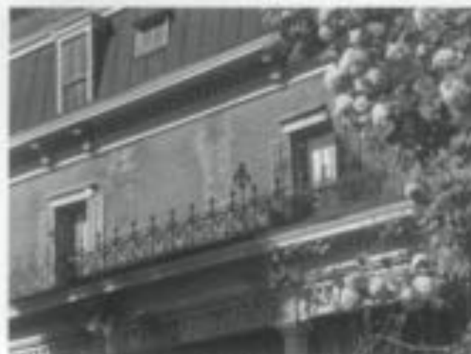
Fig. 4. Deferred maintenance often leads to blocked gutters and downspouts. This cracked gutter system allowed moisture to penetrate the upper exterior wall, erode mortar joints, and rot fascia boards. Photo: NPS files.
