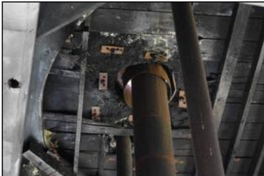
Figure 1-6: Wood infilled stack opening
