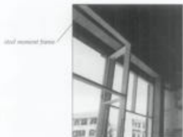
14. The use of a steel moment frame to support the large open storefront during a rehabilitation eliminated the need to place diagonal braces or other intrusive supports in a highly visible area of a historic building. Photo: David Lusk.
