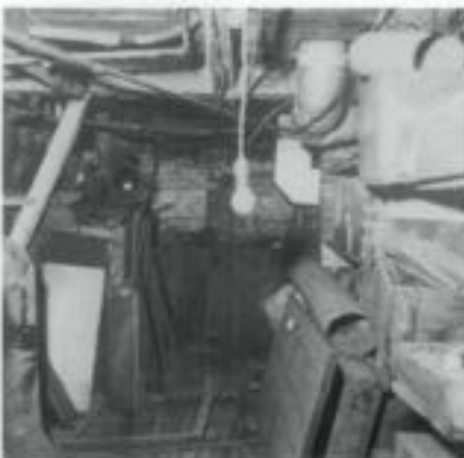
Figure F. Oxidized fixtures and systems are frequently abandoned in place when more modern units are installed. Examining and documenting their existence can provide a technological reference to the history and use of many rooms or structures. photo: NPS Preservation Assistance Division File.
