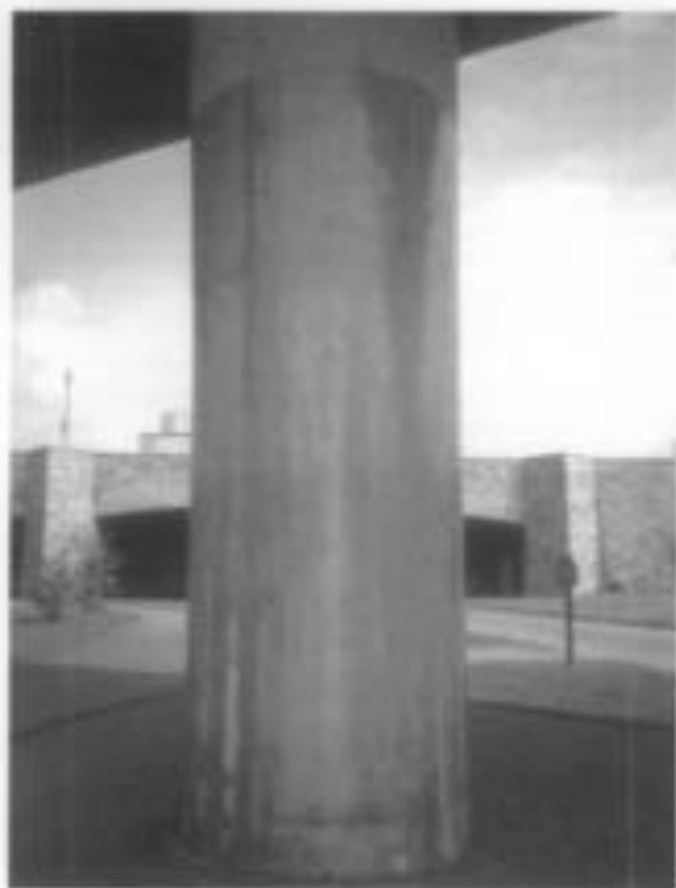
Figure 26. The anti-graffiti or barrier coating on this column is very shiny and would not be appropriate to use on a historic masonry building. The coating has discolored as it has aged and whitish streaks reveal areas of bare concrete where the coating was incompletely applied.
