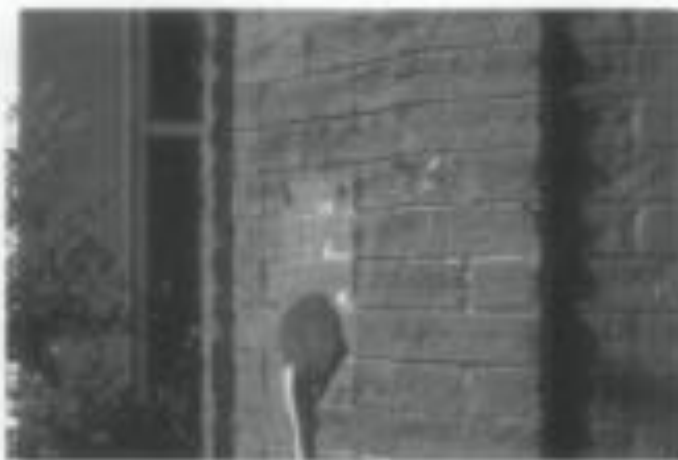
Figure 19. A comparison of undamaged bricks surrounding the electrical conduit with the rest of the brick facade emphasizing the severity of the erosion caused by sandblasting.
