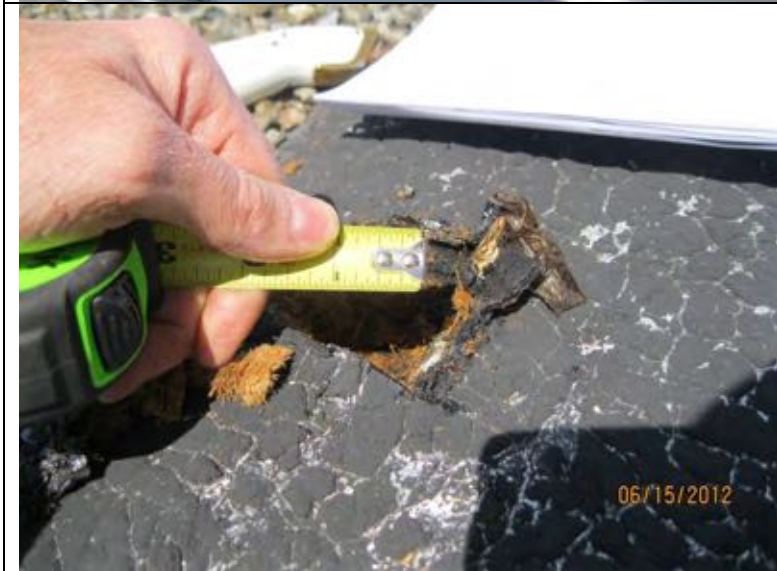
Photograph 12: Test cut at the perimeter edge of the stairwell roof confirms that the 1967 drawings appear to be accurate at the embedded metal edges.
