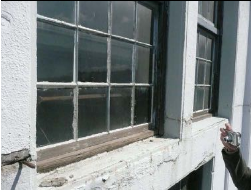
Figure 73: Detail showing existing window sill retrofits. The foreground window has a cementitious cant at the edge of the wood sill, and the background window has a newer sloped sill, which butts into the leading edge of the wood sill.
