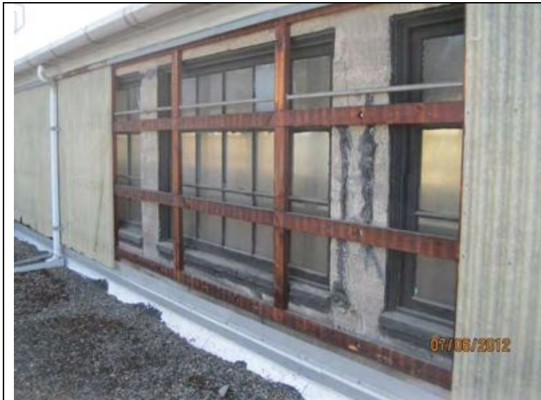
Photo 62: Clerestory wood framed windows at roof. Uncovered for condition evaluation. Note wood framing to support corrugated fiberglass is bolted to concrete. Wood sills notched in order to fit framing overlay. Wood window frames are deteriorated.
