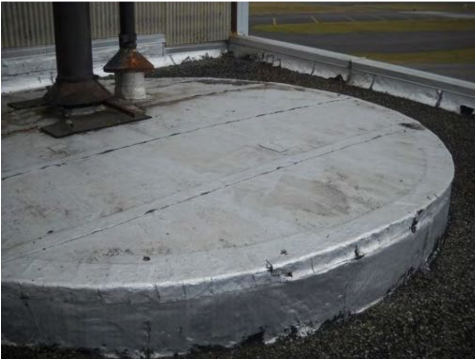
Photograph 14. RF-14: Multiple layers of silver foil over black built-up roofing and brown/pink sandy material (M)
