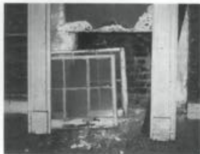
Figure 5. Loose or detached elements should be identified, tagged and stored, preferably on site. Photo: NPS files.
