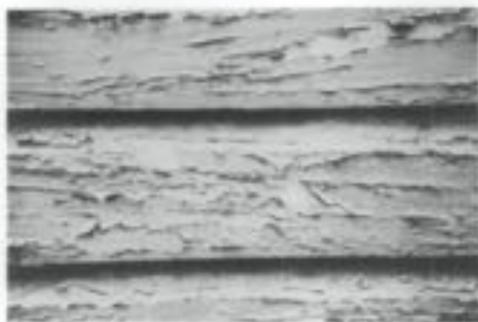
Fig. 9 Cracking, alligatoring, and flaking are evidence of long-term neglect of painted surfaces. The remaining paint on the clipboard shown here can be removed with an electric heat plate and wide-bladed scraper. In addition, unseasoned wood should be replaced and moisture problems corrected before primer and top coats of paint are applied. Photo: David W. Lock, AIA.
