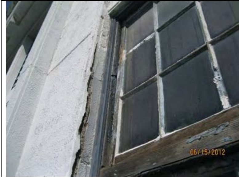
Photo 45: Spalled concrete at jamb of window, south elevation.
