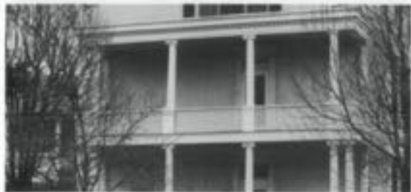
Columns were repaired and a capital was replaced in epoxy on the 19th century 3 story porch. Photo: Del Cosentino
