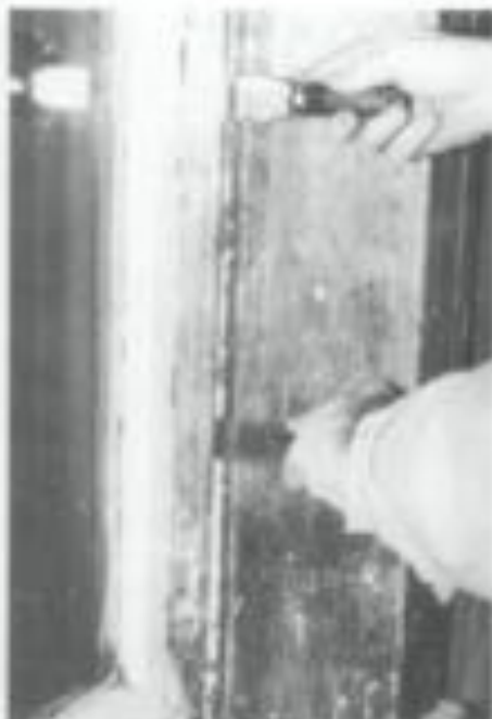
Figure 4b. After removing paint from the sash between the interior stop and the joint, the stop can be grind out and gradually worked loose using a pair of putty knives as shown. To avoid visible scarring of the wood, the sash can be raised and the stop grind loose initially from the outer side. Photo: John H. Myers
