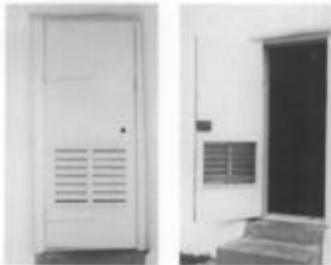
Figure 13. If historic doors would be damaged by adding extra locks, they should be removed and stored and new security doors added. At this lighthouse, the historic door has been replaced with a new door (new both inside and outside) with an inset vent and new deadbolt locks. The heavy historic hinges have not been damaged. Photo: Williamsport Preservation Training Center, NPS.
