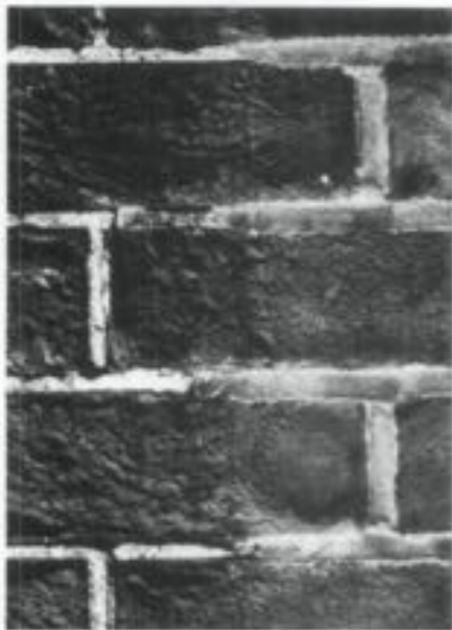
Abrusively Cleaned vs. Untouched Brick. Two brick masonry units with a common facade provide an excellent point of comparison when only one of the bricks has been sandblasted. It is clear that abrasive blasting, by removing the outer surface, has left the brickwork on the left rough and pitted, while that on the right still exhibits an undamaged and relatively smooth surface. Note that the abrasive cleaning has also removed a considerable portion of the mortar from the joints of the brick on the left side, which will require repointing.
