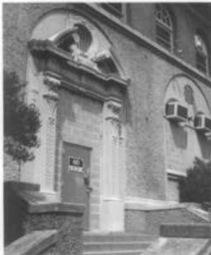
Figure 12. First floor openings have been filled with cinderblocks and doors, windows sash and frames have been removed for safe keeping. Note the security light over the windows and the use of a security metal door with heavy duty locks. Photo: H. Ward Judd, NPS.
