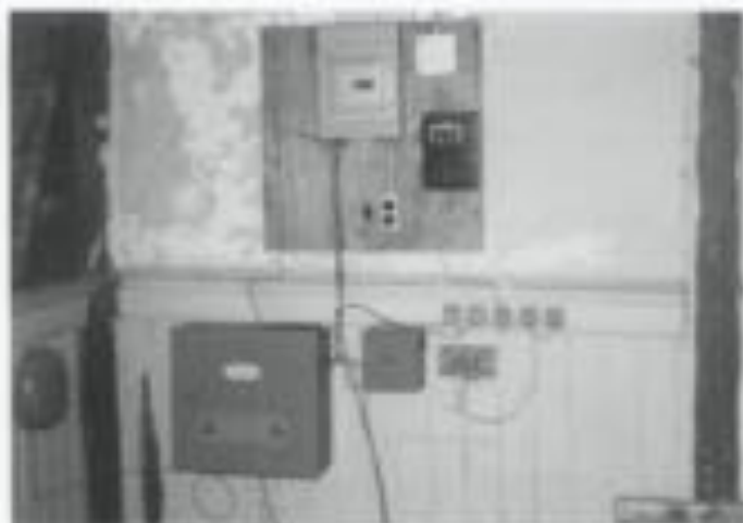
Figure 17. Security systems are very important for unstaffed buildings if they are located where fire and security services are available. A temporary electric service with battery back-up has been installed in this building. Intrusion alarms and imitation smoke/fire detectors are wired directly to the nearby security service.
