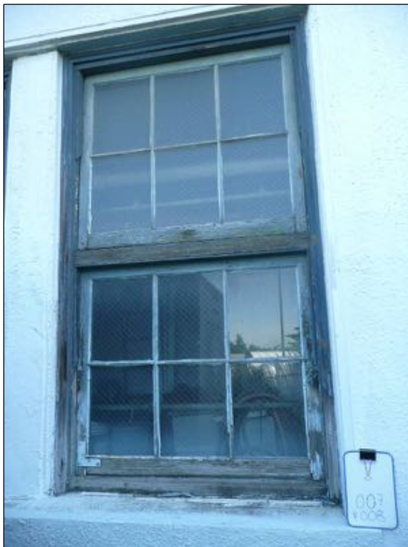
Figure 70: Detail of a window on the west facade, with little remaining paint, missing glazing, missing caulking, and previous repair at the bottom rail of the lower sash.
