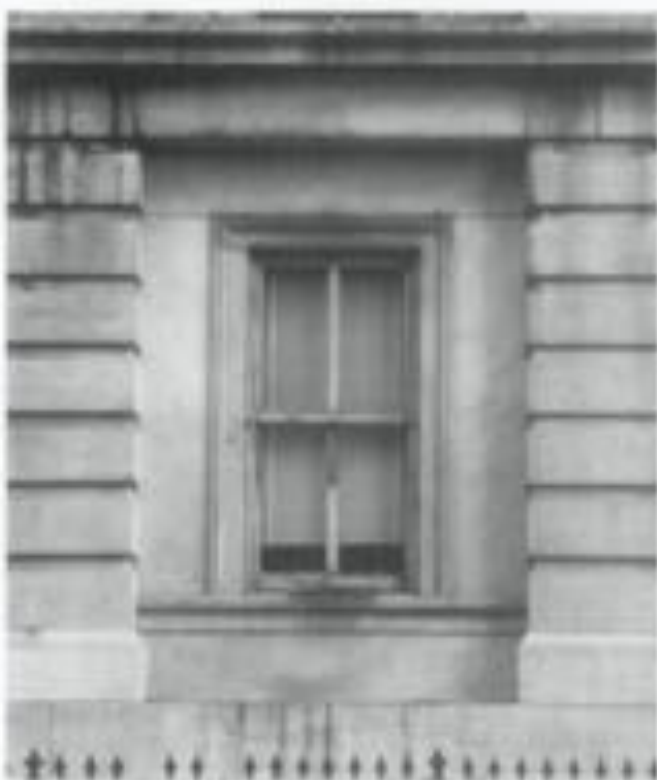
Fig. 10. Infiltration of damp air can occur around loose fitting or deteriorated window sash and through cracks or open joints in building exterior. Photo Ann Brooks Procher.
