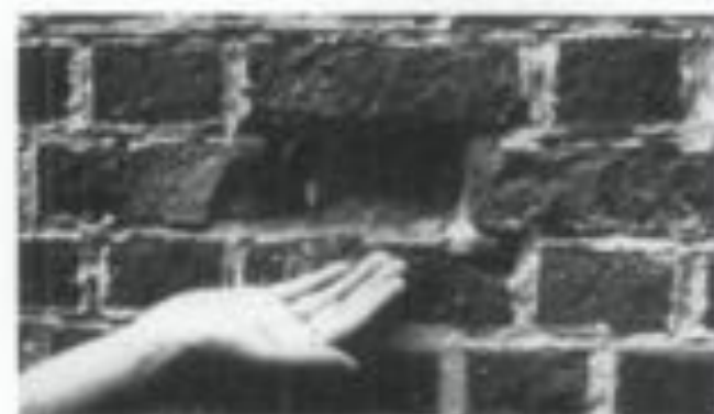
Spalling Brick. This soft, early 19th-century brick was substituted in the 1960s, consequently, severe spalling has resulted. Some bricks have almost totally disintegrated, and will eventually have to be replaced. (Robert E. Campbell)
