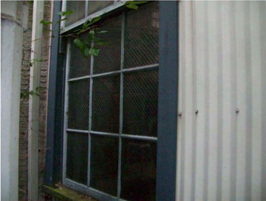
Photograph 19. HSA 15: White and grey window putty glazing for windows at far north end of east exterior (M)
