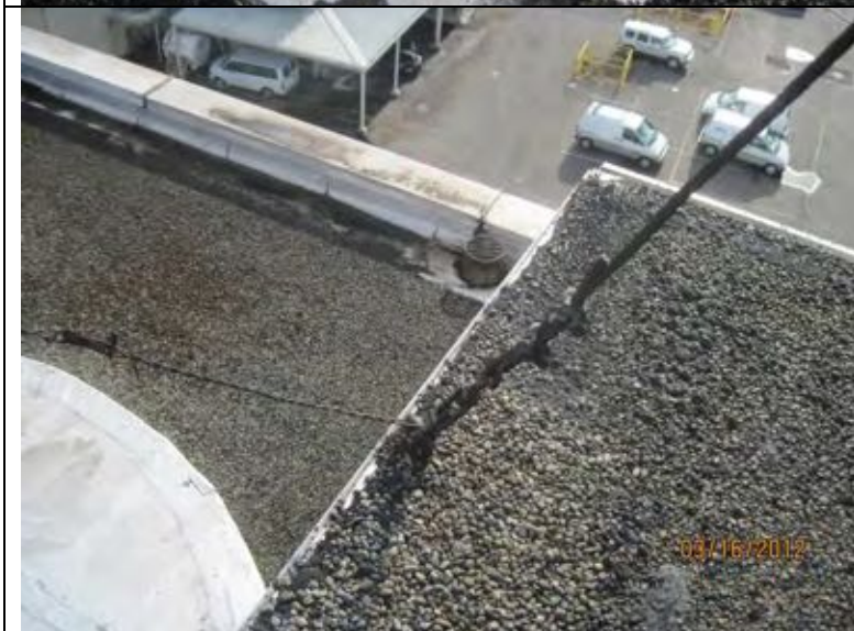
Photograph 19: Turn buckle penetration and south roof area. Guy wires are used to support stacks. Turn buckle and eyebolt penetrations need to be revised to provide a long term flashable detail.
