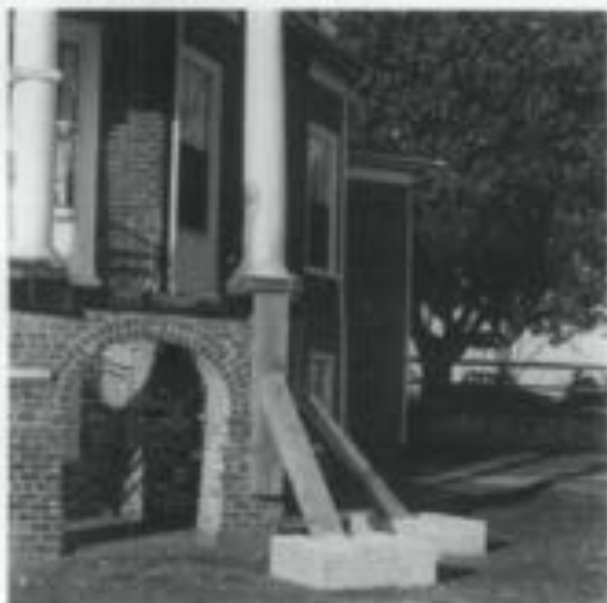
Figure 5. Investigation frequently identifies urgent needs of stabilization. Priority must be given to issues of safety and structural integrity. Supplemental support, such as temporary shoring, may be required to prevent collapse and should be reviewed by a structural engineer.
