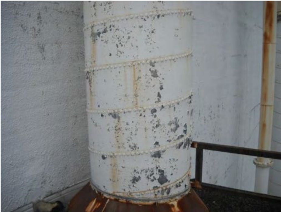
Photograph 12. RF-12: Silver paint and white/orange paint (M)
