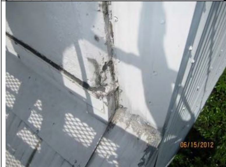
Photo 30: Corner of corrugated metal roof is not well flashed. Flashing should extend beyond corner. Sealant joint needs to be replaced or covered with sheet metal..
