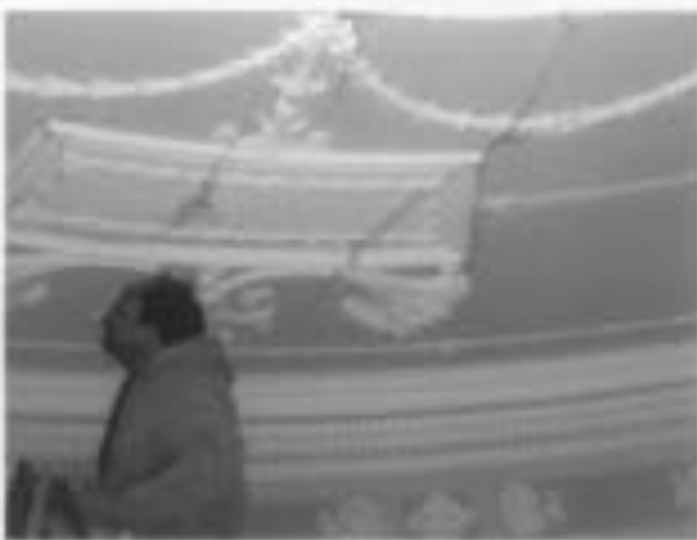
Fig. 6. Uninsulated plumbing pipes close to the exterior wall froze and cracked, setting this ornamental plaster ceiling before the water supply line could be shut off. As a result, limited portions of the ceiling needed retouching. Photo: author.
