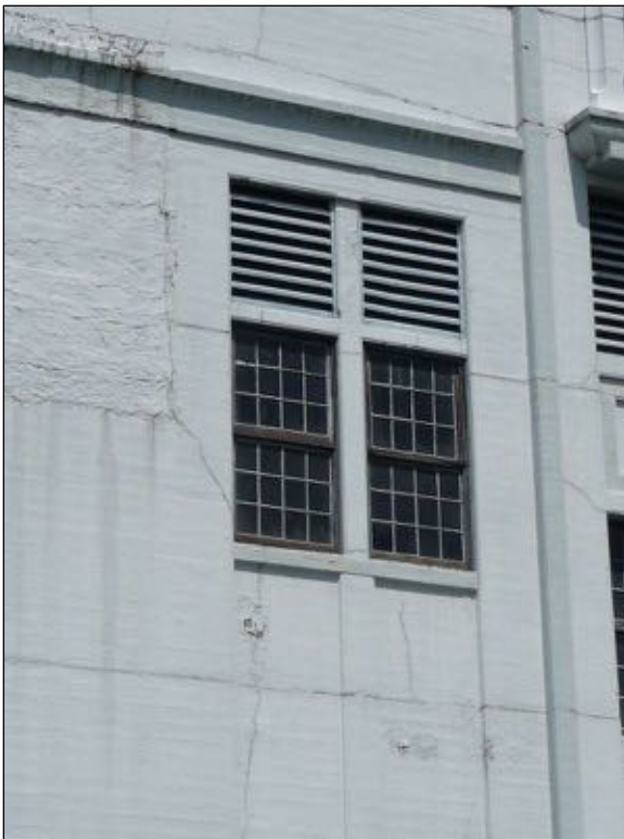
Figure 51: Detail of south wall, showing horizontal cold joints, and various cracks treated with joint sealant.
