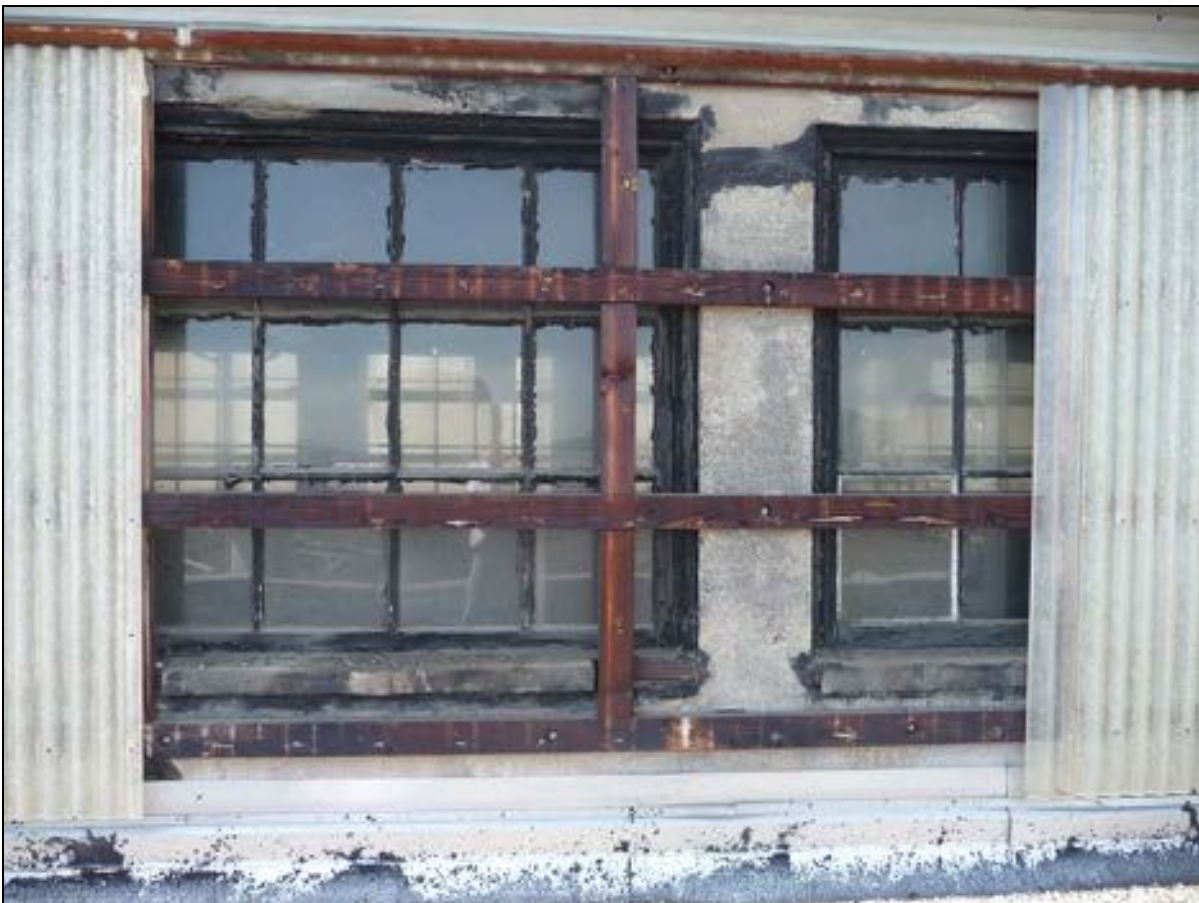
Figure 57: Detail of Engine Room monitor wall with fiberglass panels partially removed. Note the mastic patching, the wood sills notched for the fiberglass support framing, and the framing bolted into the concrete.
