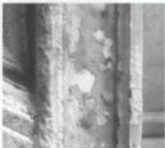
Figure 25. The clear coating applied to this limestone masonry has failed and is taking off some of the stone surface as it peels. Photo: Frances Gale.
