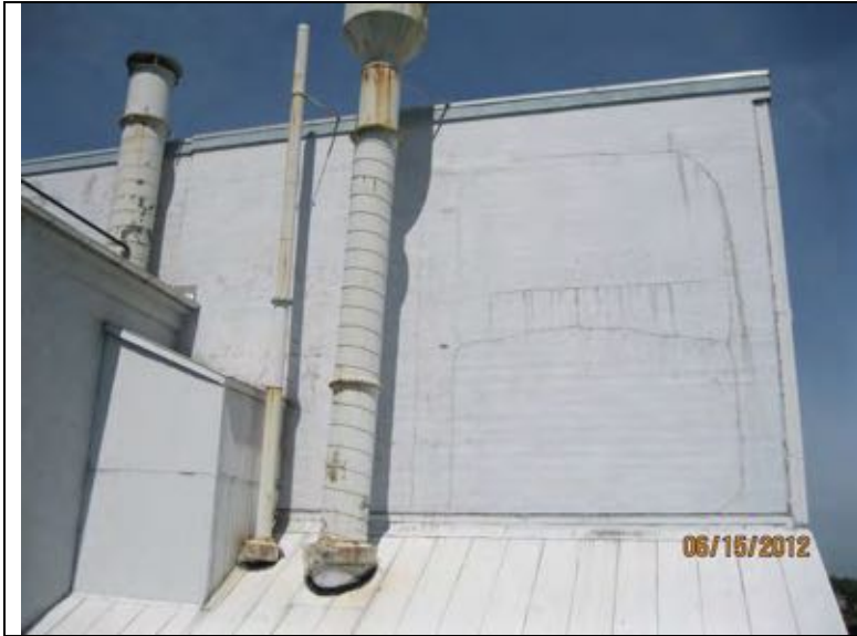
Photo 48: Overview of south facing wall at 1918 addition. This wall includes parge coat over board formed concrete.
