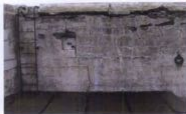
Figure 13. Fort Casey on Admiralty Head, Fort Casey, Washington, was constructed in 1888. The lift lines from placement of concrete are clearly visible on the exterior walls and characterize the finished appearance.
