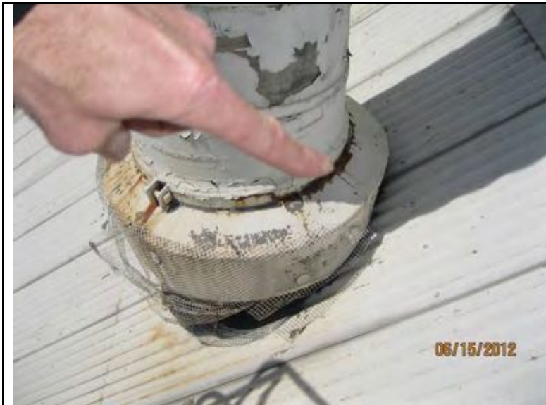
Photo 32: Pointing out where flashing is rusted through.
