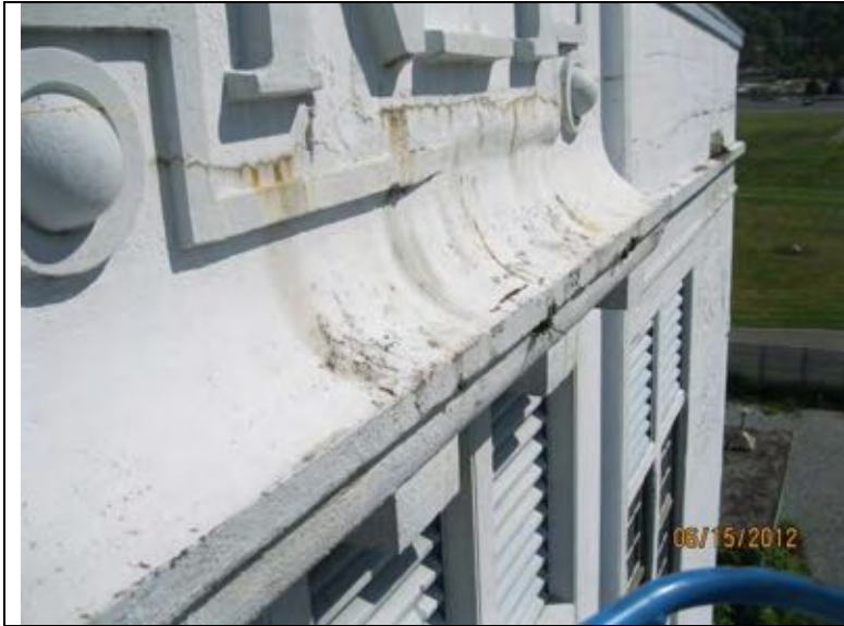
Photo 42: South elevation with station label. Note inaccurate patching at wall and cracks/spalls where water has caused plant growth at drip edge.
