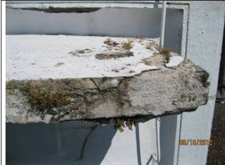
Photo 43: Spalled and delaminated concrete at corner of cornice, south elevation top of wall.
