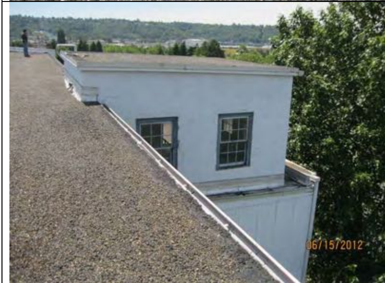
Photograph 9: Overview of north stairwell roof and roof areas below that wrap around the stairwell roof.
