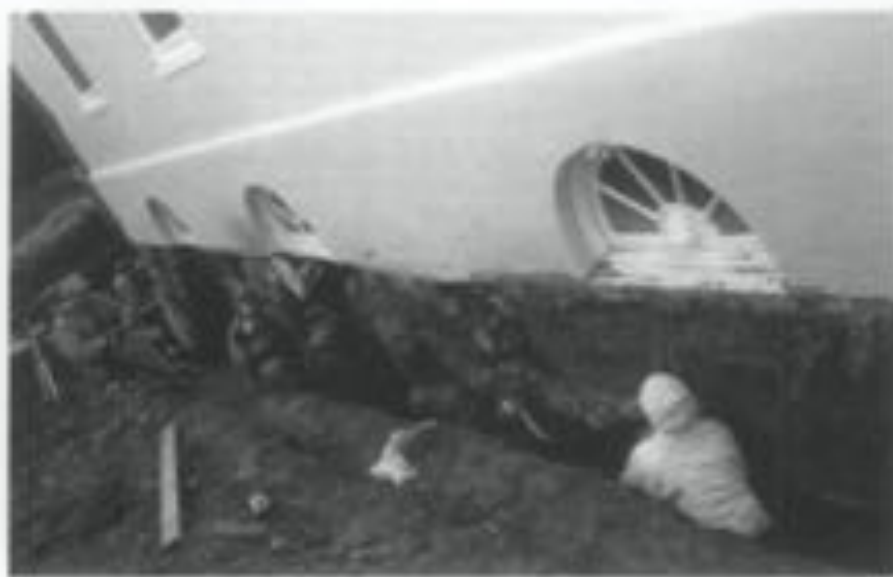
I. Critically damp foundation walls were protected with a layer of bentonite clay to reduce moisture penetration. This work was in combination with new drainage pits that were connected to drainage basins that deposited captured roof run-off away from the foundation. Photo: Courtesy, Larry D. Dornosky and the National Trust for Historic Preservation.
