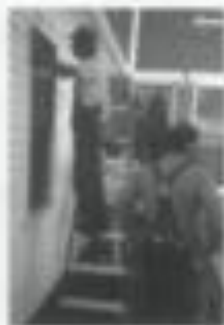
B. Repair exterior surfaces, paint, and caulk as needed. Photo: Williamsport Preservation Training Center (WPTC), NPS.
