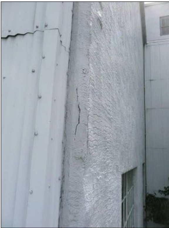
Figure 61: Detail of northeast corner of the 1918 Addition, with corrugated metal and stucco-clad hollow clay tile. Delamination of the stucco is evident at the corner.
