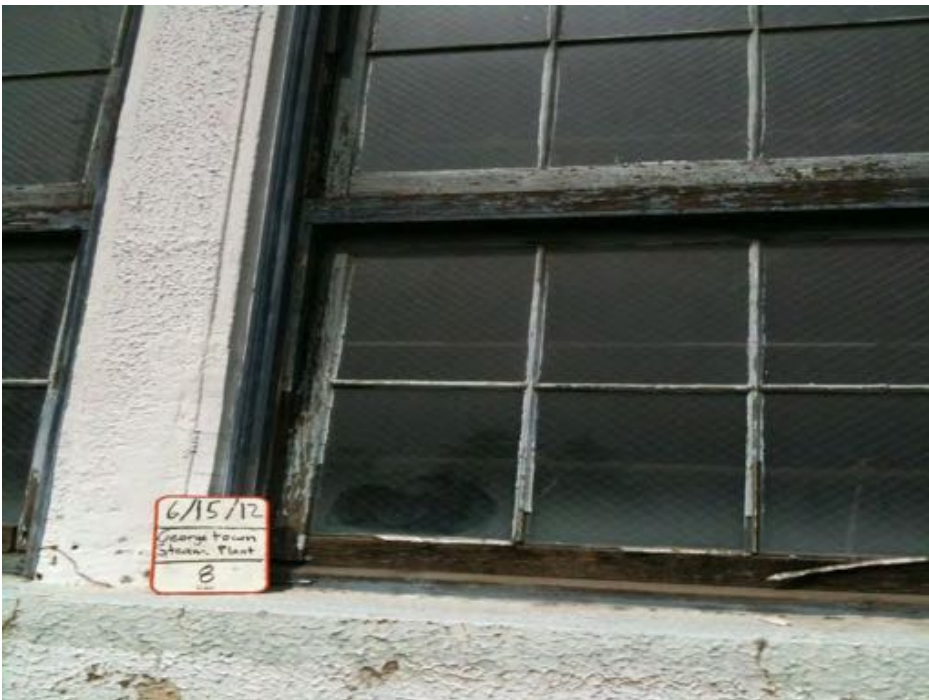
Photograph 12. HSA 8: Beige/grey window putty glazing (M)
