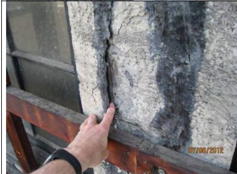
Photo 63: Severely spalled concrete and exposed/rusted reinforcing steel.
