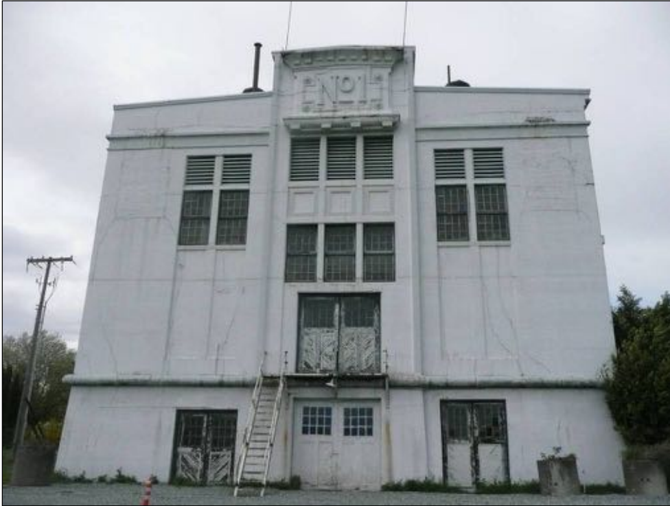
Figure 50: South façade, showing significant cracking throughout the wall areas.
