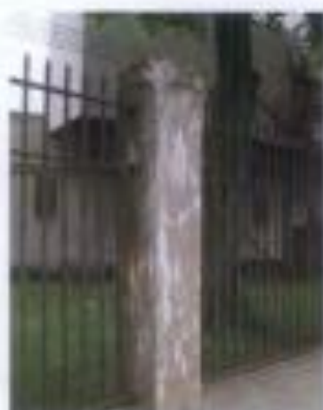
Figure 15. Evidence of moisture movement through concrete is apparent in the form of mineral deposits on the concrete surface. Cyclic freezing and thawing of entrapped moisture, and corrosion of embedded reinforcement, have also contributed to deterioration of the concrete columns on this fence at Crocker Field in Fitchburg, Massachusetts, designed by the Olmsted Brothers.
