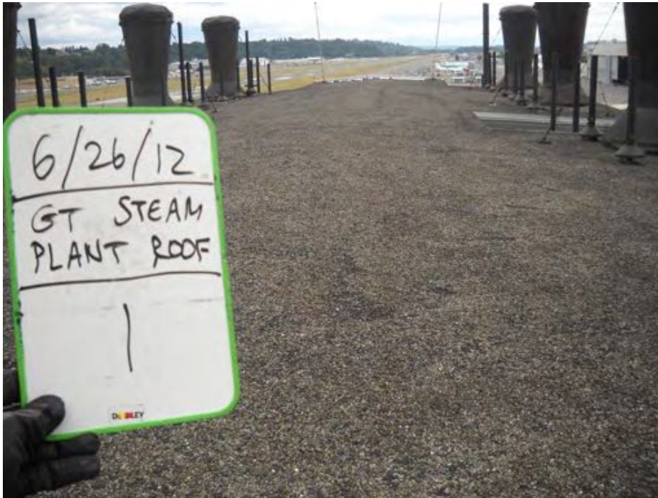
Photograph 1. RF-1: Multi-layer black built-up roofing with pebbles, black asphaltic sealant and black fibrous material (M)
