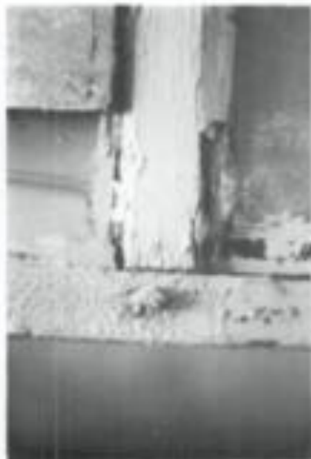
Figure 4a. The following series of photographs of the repair of a historic double-hung window use a sash which is structurally sound but has many layers of paint, some cracked and missing putty, slight separation at the joints, broken sash cords, and one cracked pane. Photo: John H. Myers
