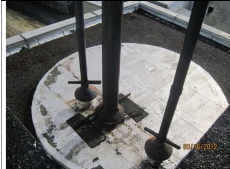
Photograph 18: Circular roof with KMM membrane at SW corner. We understand from 1983 drawings this is the original stack through the roof and the raised portion is a wood framed cover that has been roofed and flashed into the gravel surfaced roof.
