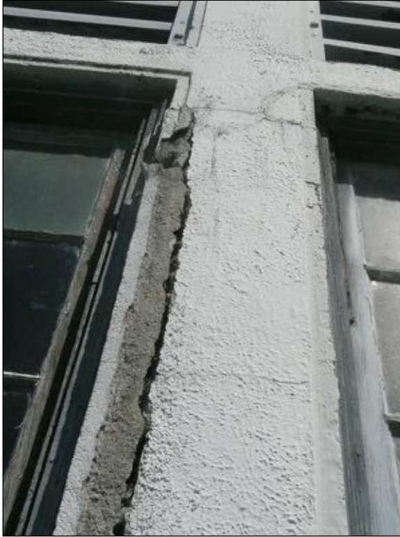
Figure 53: Detail of windows on the south wall. The concrete mullion is cracked and delaminating about an inch from the face of the wall.
