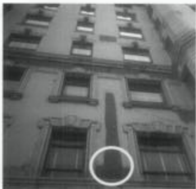
Figure 3. This small test area has revealed a red brick patch that does not match the original large brick. This may explain why the building was painted, and may suggest to the owner that it may be preferable to keep it painted.
