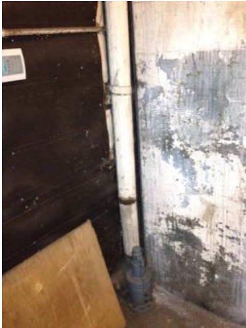
Image 7: East side Boiler Rm drain pipe
