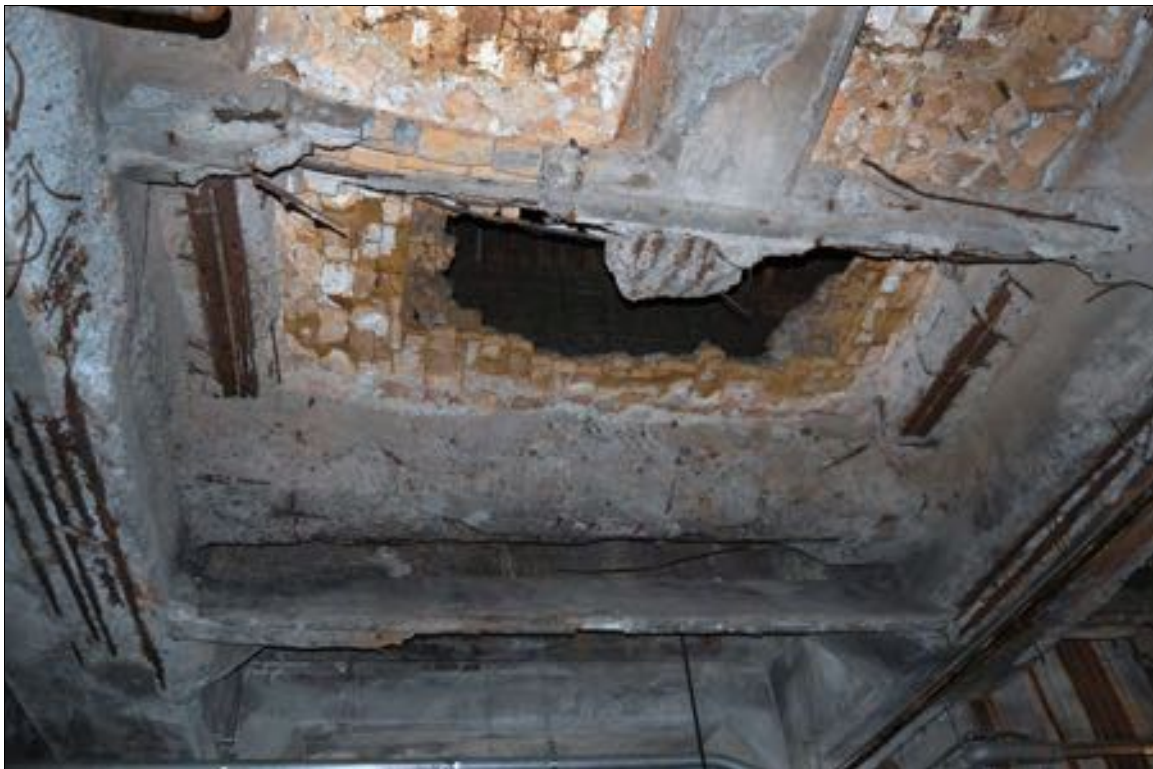
Figure 3. Damage resulting from demolition of ash hopper.
