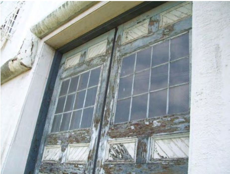
Photograph 20. HSA 16: Beige window putty glazing with paint on windows for wood doors at north end of west exterior (M)
