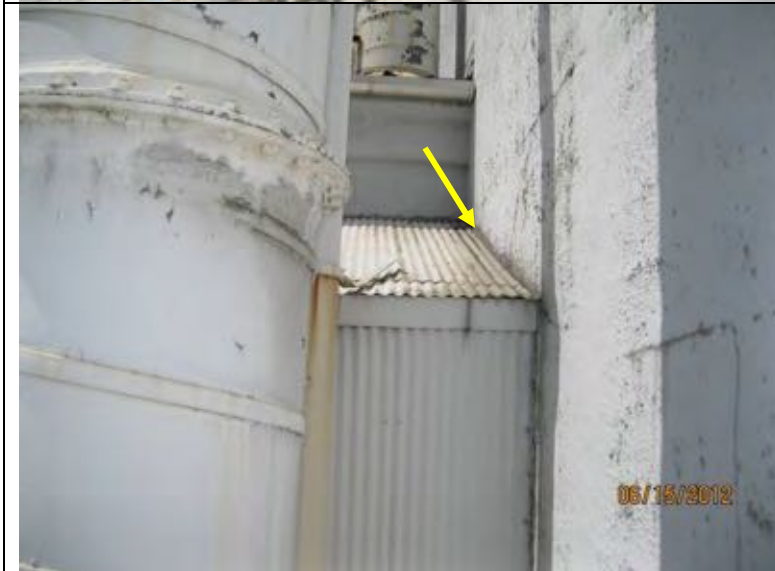
Photo 33: Upper corrugated metal roof drains to lower metal roof. There is no counterflashing along the rake edge of the upper roof. It appears the roofing butts to the wall.
