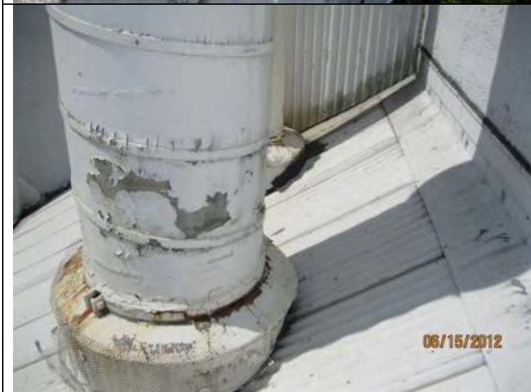
Photo 31: Stack penetrations through corrugated metal roof need to be reflashed and sealed, as the metal flashing is rusted through in locations.
