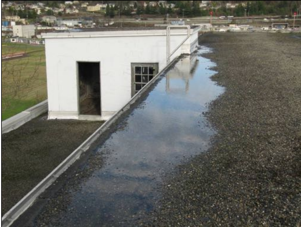
Figure 65: Detail of water ponding in the shallow swale at the edge of the embedded metal eave flashing, atop the Engine Room monitor roof.
