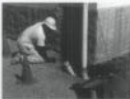
C. Cleaning out gutters and downspouts should be done at least twice a year. Photo: WPTC, NPS.
