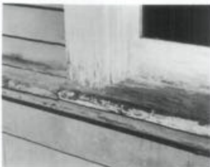
Fig. 4 Paint film wear unevenly depending on exposure and location. Exterior locations which are susceptible to accelerated deterioration are horizontal surfaces such as window sills. These and similar areas will require repainting more often than less vulnerable surfaces. In the case of this window sill where paint has peeled off and adjacent areas have cracked and alligatored, the paint should be totally removed. Prior to repainting, any weathered wood should be rejuvenated using a solution of 2 cups exterior varnish, 1 oz. paraffin wax, and mineral spirits/paint thinner/or turpentine to make 1 gallon. Liberal brush application should be made. This formula was tested over a 20-year period by the U.S. Department of Agriculture's Forest Products Laboratory and proved to be just as effective as water-repellent preservatives containing pentachlorophenol. After the surface has thoroughly dried (2-3 days of warm weather), the treated surface can be painted. A high quality oil-base primer followed by two top coats of a semi-gloss oil-m enamel or latex-m enamel paint is recommended. Photo: Beird M. Smith, AIA.
