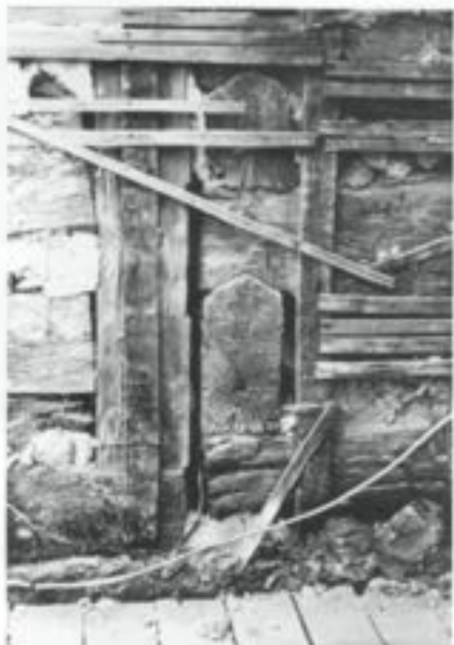
Fig. 8. Removal of deteriorated stucco in preparation for stucco repair on this late-19th century log house in Middleway, West Virginia, reveals that the stucco was applied to hand-riven wood lath nailed over vertical wood strips attached to the logs. Photo: Anne Grimmer.
