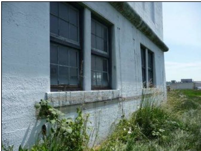
Figure 48: Example of vegetation on the building, biological growth and surface staining and deterioration.
