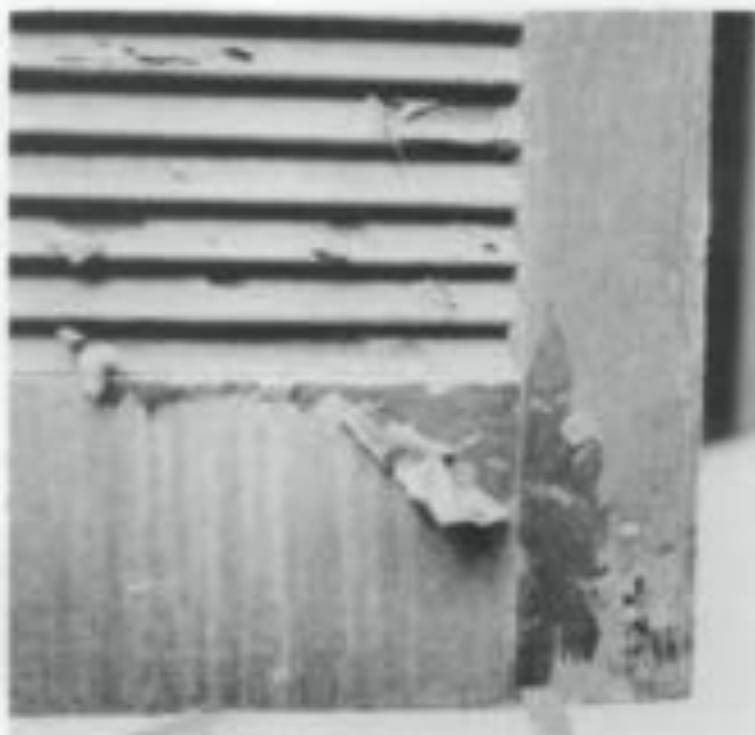
Fig. 6 This is an example of intercoat peeling. A latex top coat was applied directly over old oil paint and, as a result, the latex paint was unable to adhere. If latex is being used over oil, an oil base primer should be applied first. Although much of the peeling latex paint can be scraped off, in this case, the best solution may be to chemically strip the entire shutter to remove all of the paint down to bare wood, rinse thoroughly, then repaint. Photo: Mary L. Dehelen, AIA.
