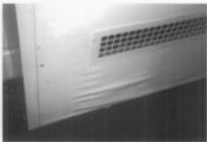
Fig. 3. The deterioration of this vent cover was a sign that water was leaking from the fan coil unit behind. Photo: author.
