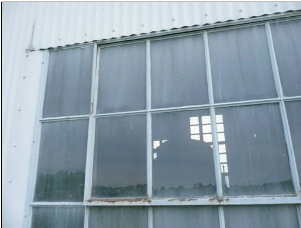
Figure 60: Detail of lapped flashing at steel window depends on caulk for water protection.
