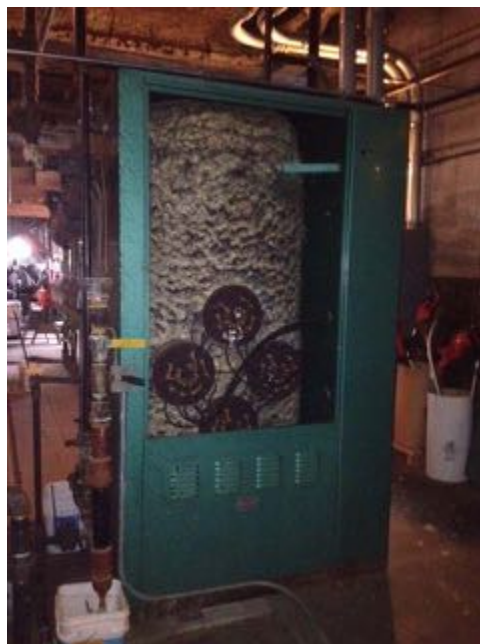
Image 10: Boiler access panel removed
