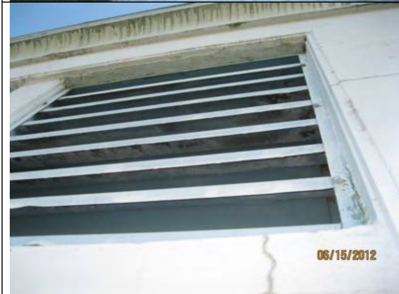
Photo 41: Steel louvers at top of west elevation appear to be in serviceable condition, other than surface preparation and paint.
