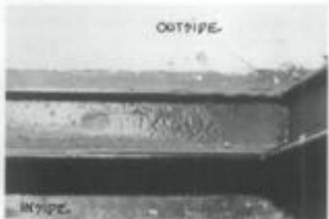
Fig. 6 e. View looking down towards the sill. The cleaned frame was reset in the window opening. The frame was screwed to the refurbished subframe at the jamb and the head only. The screw holes at the sill, which had been the cause of much of the earlier rusting, were infilled. Vinyl weatherstripping was added to the frame.
