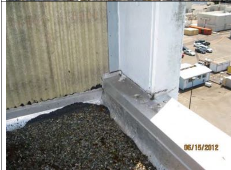
Photograph 5: Coping to wall at the NW roof. The coping is not sufficiently counterflushed.
