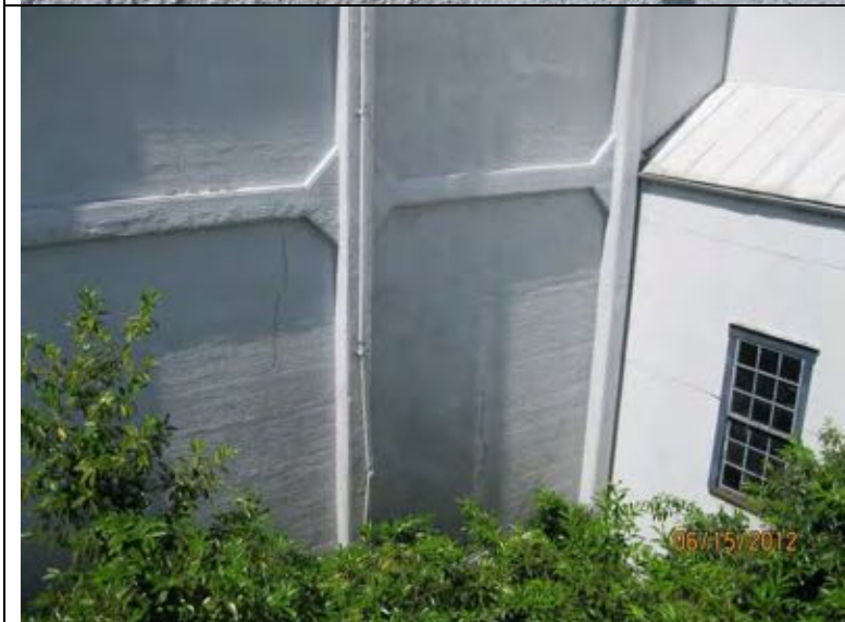
Photo 47: Overview of a portion of the east elevation south of the Engine Room.
