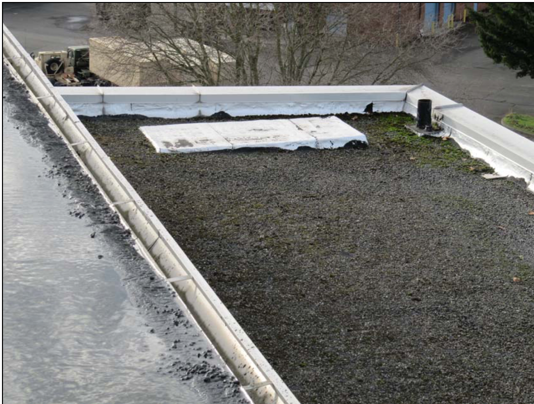
Figure 63: Detail showing the “low profile” eave gutter roof at the Engine Room monitor roof at left, and the raised profile of the parapet at the northwest corner of the Engine Room at right.
