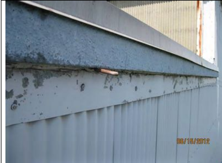
Photo 52: Sheet metal wall panels appear to butt to underside of concrete at east end of engine room roof. Sealant knife is inserted in open joint.
