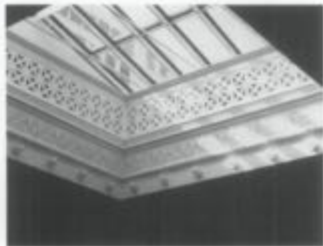
7. Operable skylights and grilles that can be adapted for where air should be identified as part of the planning phase for new or upgraded mechanical systems. Photo: Damon Pierce, NPS files
