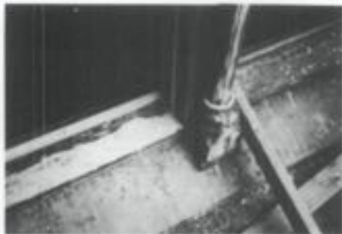
Illus. 7. Whenever possible, historic materials should be repaired rather than replaced. Epoxy, a synthetic resin, has been used to repair the wood window frame and sill at the Auditors Building (1878) Washington, DC. The cured resin is white in this photo and will be ground and painted. Photo: Lee H. Nelson, FAIA.
