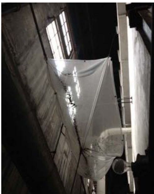
Image 5: West side Boiler Room leak
