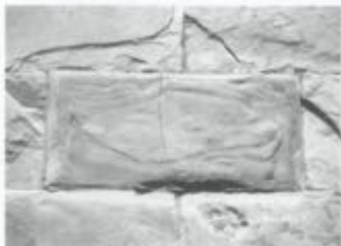
Illus. 19. When the physical properties are not matched, particularly thermal expansion and contraction properties, great damage can occur. In this case, an extremely rigid epoxy replacement unit was installed in a historic masonry wall. Because the epoxy was not modified with fillers, it did not expand or contract systematically with the natural stones in the wall surrounding it. Pressure built up resulting in a vertical crack at the center of the unit, and spalled edges to every historic stone that was adjacent to the rigid unit. Photo: Walter M. Sorethamer.
