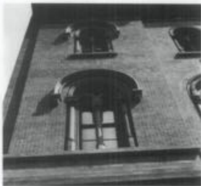
Illus. 8. Even when materials are not locally available, it may be possible and cost effective to find sources elsewhere. For example, the local sandstone was no longer available for the restoration of the New York Shakespeare Festival Public Theater. The deteriorated sandstone window heads were replaced with stone from Germany that closely matched the color and texture of the historic sandstone. Photo: John G. Waite.
