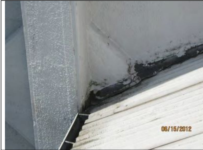
Photo 35: Close-up of previous photo at bottom edge (SW corner of roof). This is a built in leak where the roofing runs into a concrete column. There needs to be a custom soldered cricket/diverter installed with counterflashing on the wall.
