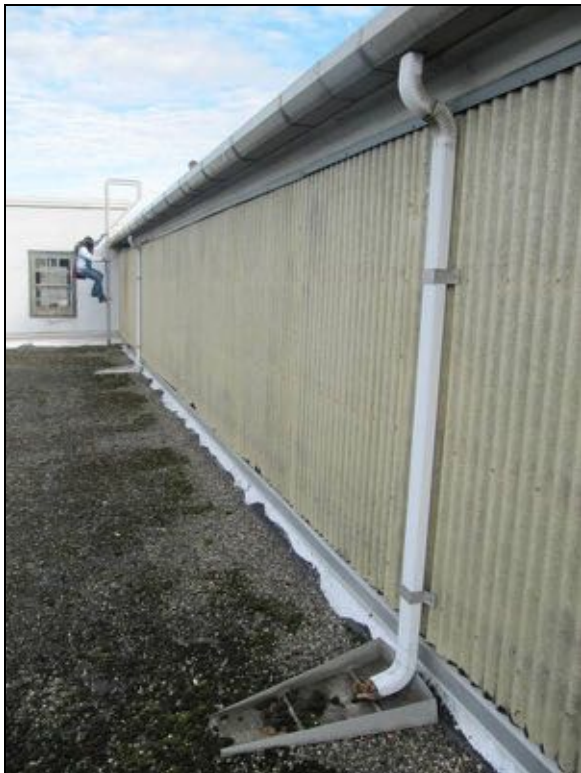
Figure 64: Typical roof monitor downspout and splash block draining onto the main Engine Room roof.
