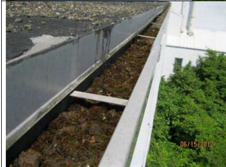
Photo 27: Gutter is full of debris indicating maintenance is not performed, at least to clean gutters.
