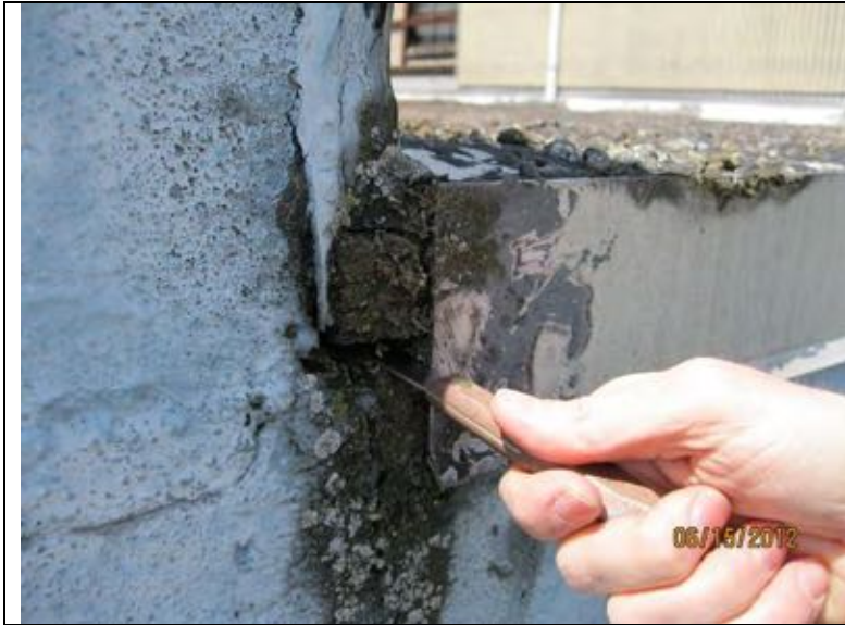
Photo 51: Edge of low slope roof without closure where embedded edge metal meets parapet wall. Wood nailer below metal flashing is exposed. Photo taken at east end of south engine room roof.
