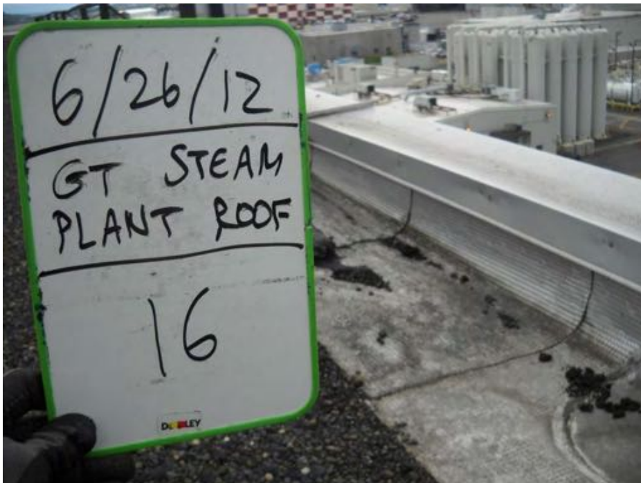
Photograph 16. RF-16: Silver foil over black built-up roofing over black asphaltic sealant over black felt (M)
