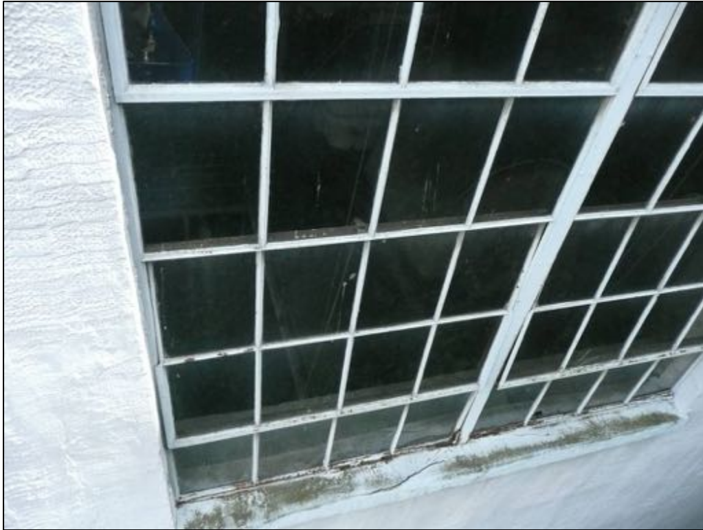
Figure 77: Detail of a steel window, with rust on the frame at the bottom, and a cracked concrete sill.
