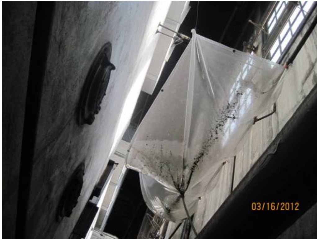
Figure 66: Roof drain leak catcher at the west side of the Boiler Room (photo by Wetherholt and Associates)
