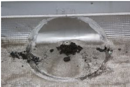
Image 3: Existing roof drain
