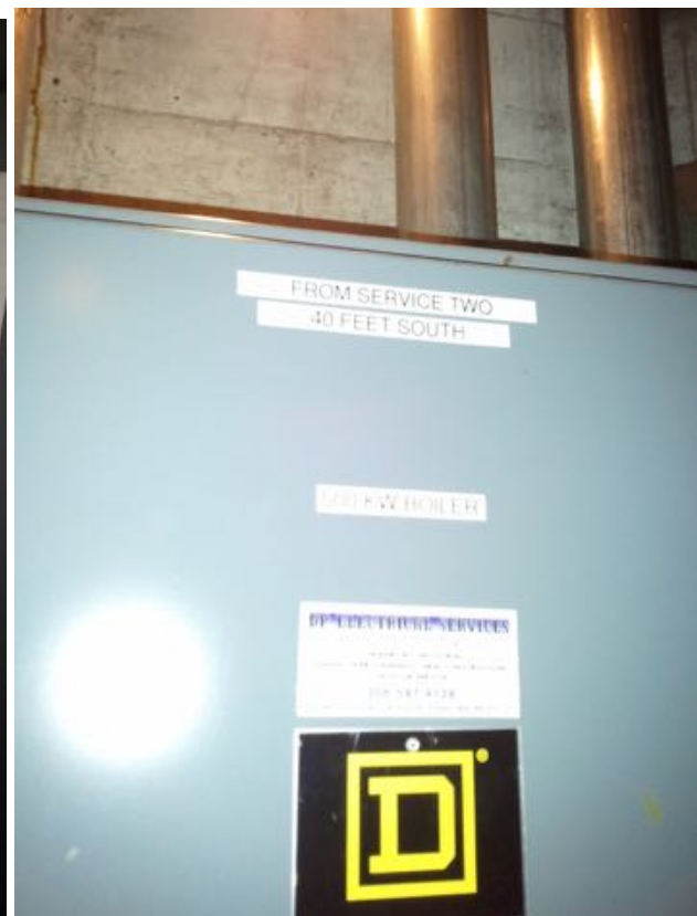
Image 2: 500kW Boiler Disconnect
