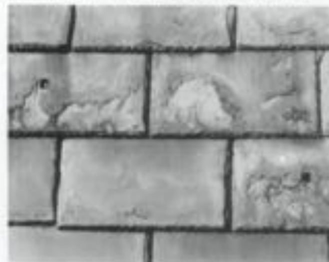
This detail shows slate delamination caused by a combination of weathering and pollution. In addition, the slates have eroded around the repair nails, incorrectly placed in the exposed surface of the slates (Lower Pontalba Building, New Orleans, photo courtesy of Building Conservation Technology, Inc.)
