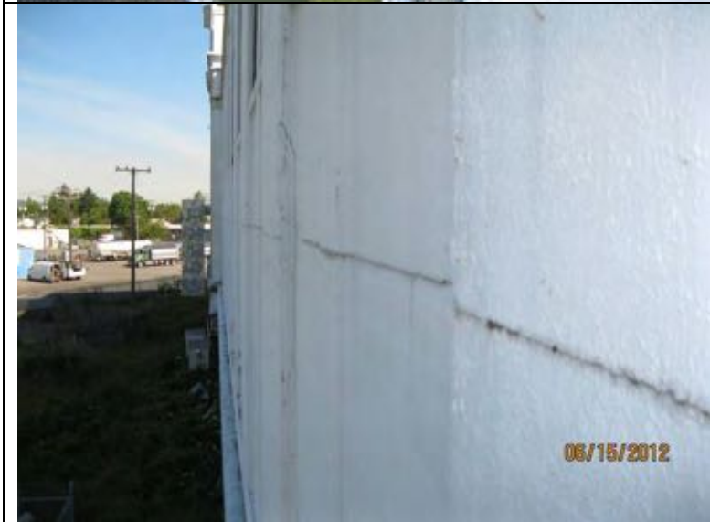
Photo 38: Horizontal crack in what appears to be a cold joint in the concrete at the west elevation.
