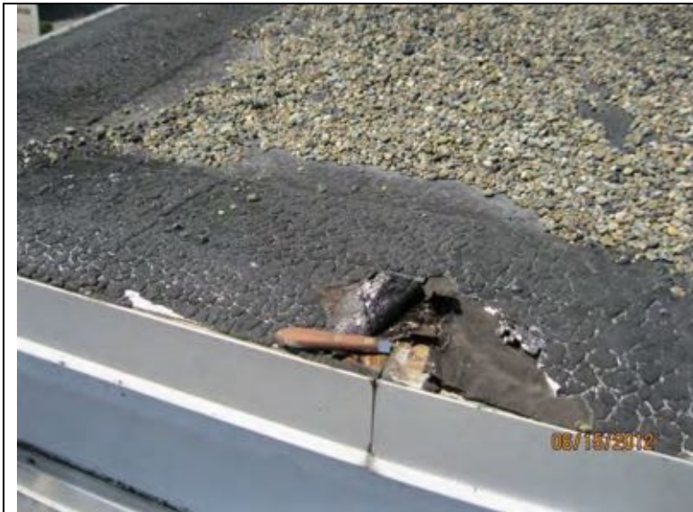
Photograph 11: Membrane unadhered and peeling from edge metal at lap joint in edge metal. Note sealant knife is inserted under the edge metal, which does not appear to be sealed in the lap joint.
