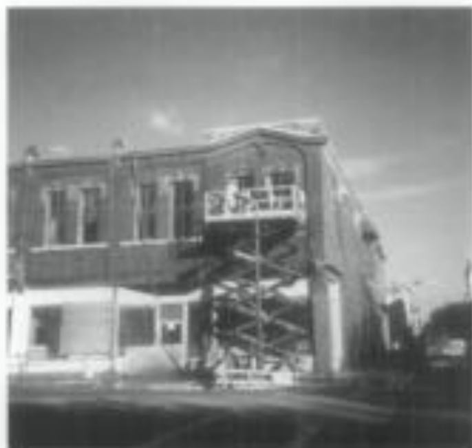
Figure 14. Chemical removal of paint from this brick building has revealed that the cornice and window heads are metal rather than masonry.
