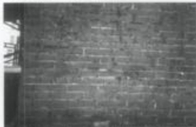
Figure 13. Sometimes it may be preferable to paint over a thick asphalt coating rather than try to remove it, because it can be difficult to remove completely. However, in this case, many layers of asphaltic coating were removed through multiple applications of a heavy duty chemical cleaner. Each application of the cleaner was left to dwell following the manufacturer's recommendations, and then rinsed thoroughly. (As much as possible of the asphalt was first removed with wooden scrapers.) Although not all the asphalt was removed, this was determined to be an acceptable level of cleanliness for the project.
