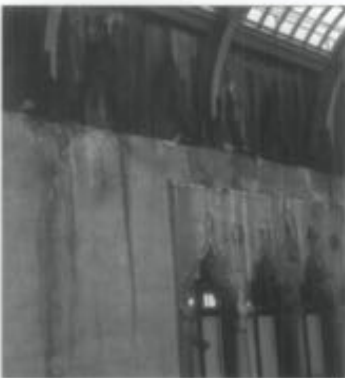
Fig. 7. Condensation dripping from the large overhead courtyard skylight was damaging the masonry in this museum. A new skylight with thermal glazing was installed, replacing the deteriorated single-glazed unit. A new climate control system maintains interior temperature and humidity. Photo © Judith Stewart Gardner Museum, Boston.
