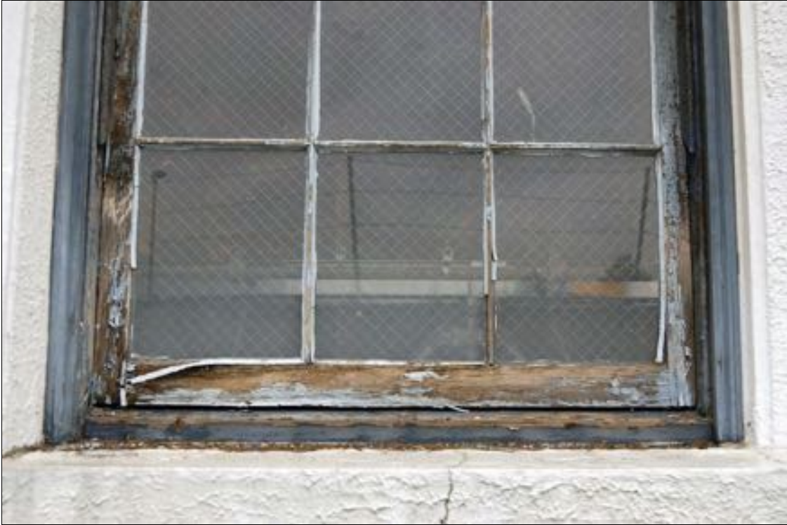
Figure 7. Detail of weathering and deterioration of southwest-facing window, view to the northeast.
