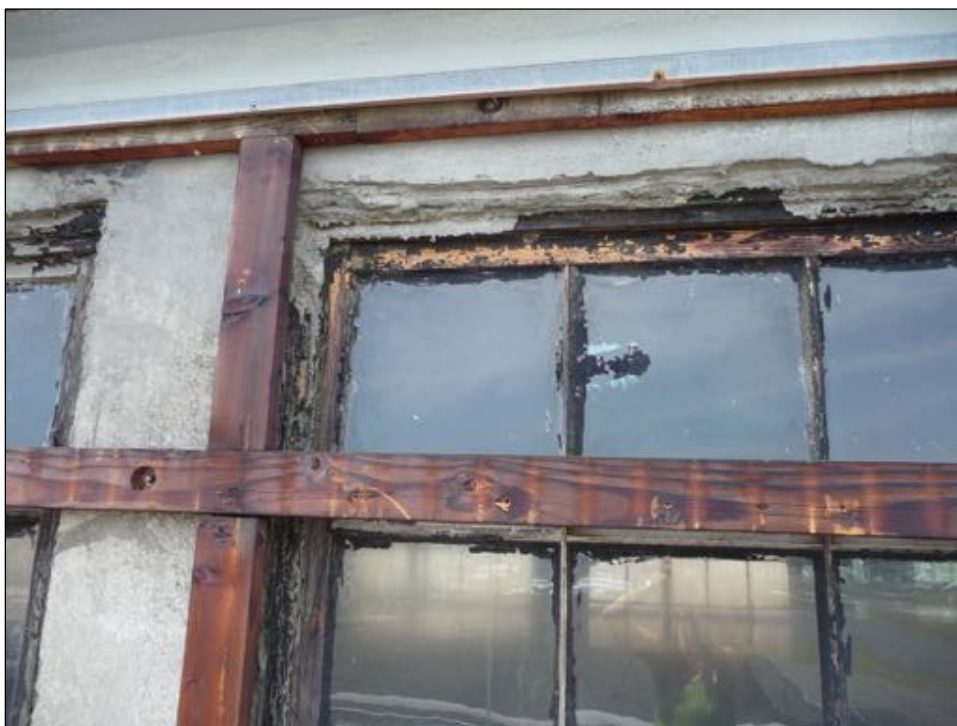
Figure 75: Some monitor window sills retain their original lead covers. In some instances, the wood sills and lead covers were notched or sawn off entirely in order to install the wood framing for the protective fiberglass panels.
