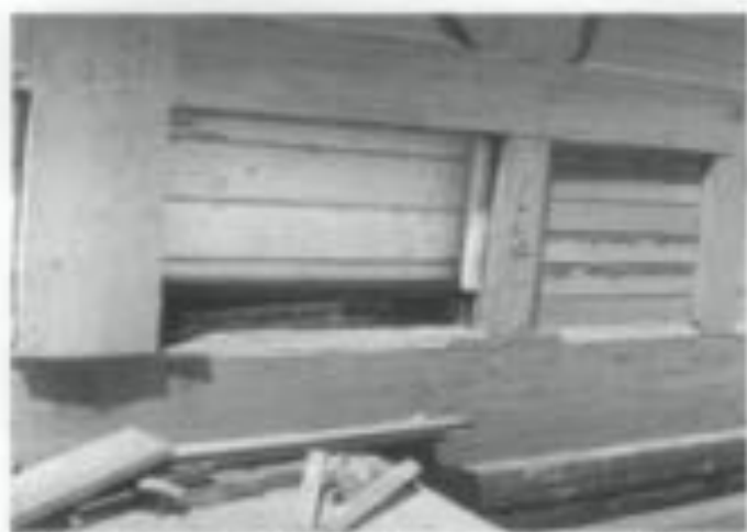
Fig. 8. Damaging moisture conditions can occur during construction. Peeling paint on this newly rehabilitated frame wall was attributed to wall insulation that had become wet during the project and was not discovered. Photo: NPS Files.
