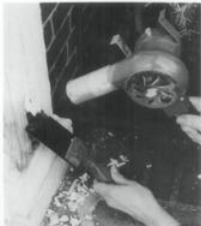
Fig. 24. The nozzle on the electric heat gun permits hot air to be aimed into cavities on solid decorative elements such as this applied column. After the paint has been sufficiently softened, it can be removed with a profiled scraper. Photo: Charles E. Fisher, III.
