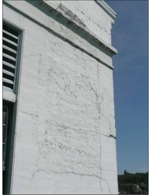
Figure 54: Detail of east arched opening infill on the south wall, with mismatched texture.
