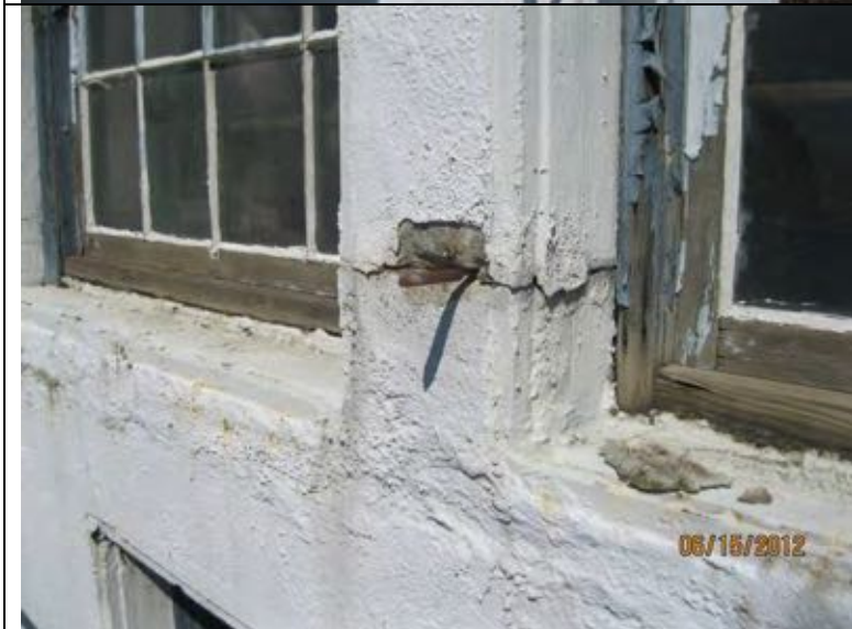
Photo 44: Sealant knife inserted into what appears to be an open cold joint in the concrete between windows, south elevation.
