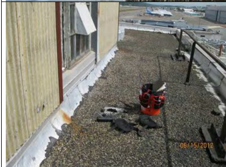
Photograph 25: Test cut at south end of south roof, west side. Similar to previous test cuts.
