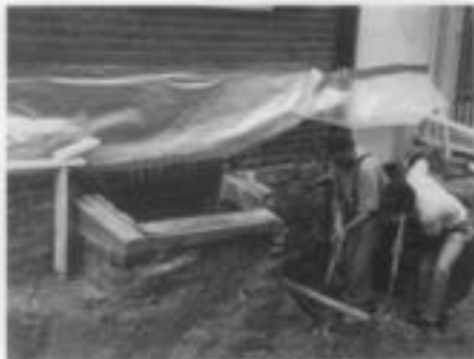
Fig. 5. Excavating this foundation revealed that the downspout pipe had corroded at the "u-trap" and was leaking moisture into the soil. Openings around the horizontal water supply line and cracks in the wall allowed moisture to penetrate the basement in multiple locations. Photo: author.
