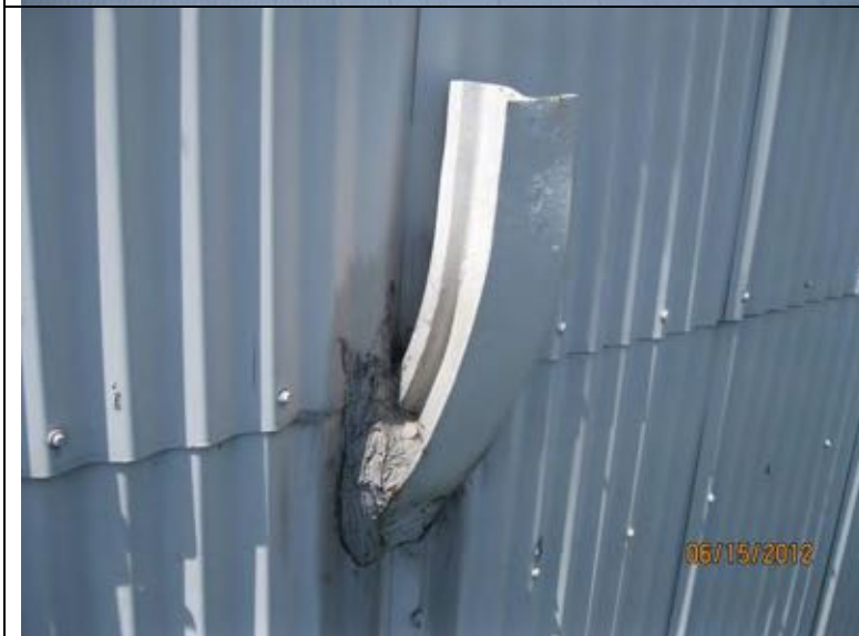
Photo 50: Rail tracks extend through siding and are bent up. Sealant applied around penetrations is not watertight.
