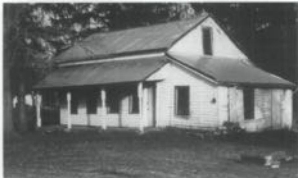
Figure 7. Non-historic materials are appropriate for mothballing projects when they are used to protect historic evidence remaining for future preservation. This lightweight aluminum channel frame and roofing covers the historic wooden shingle roof. Galvanized mesh panels across the window openings protect from intrusion by raccoons and other unwanted guests. Photo: Williamsport Preservation Training Center, NPS.
