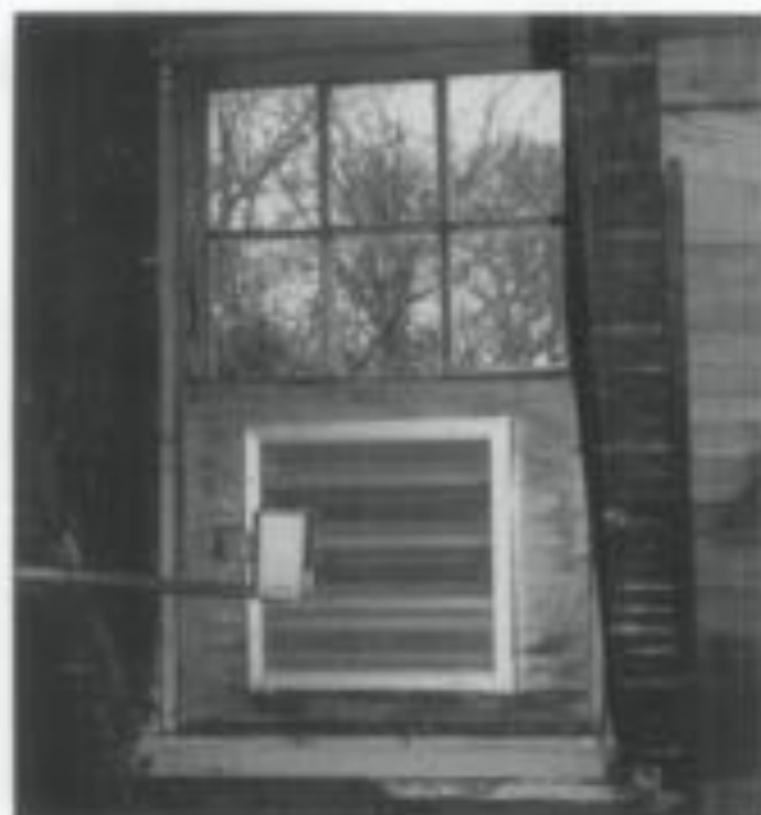
Figure 21. This electric thermostat/humidistat mounted in the attic zone controls a modified ducted air/fan system. The unit uses temporary expandable metal ducts to pull air through the building and exhaust it out of the basement. For over ten years this fan system in combination with 18" x 28" professional louvers in selective windows has kept the interior dry and with good air exchange.
