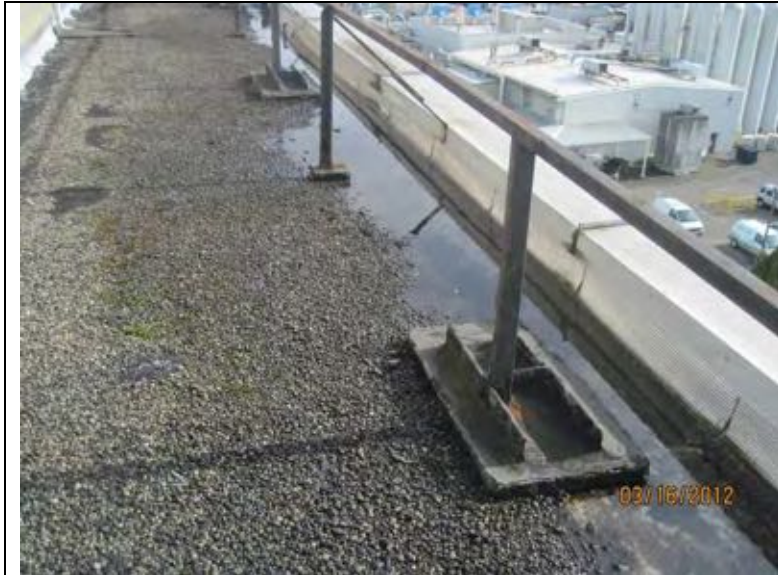
Photograph 23: Handrails on east and west sides of the roof are apparently welded to steel angles bolted to the roof substrate. Pitch pockets are placed around the angles. These penetrations need to be revised to round pipe penetrations that can be properly flashed.
