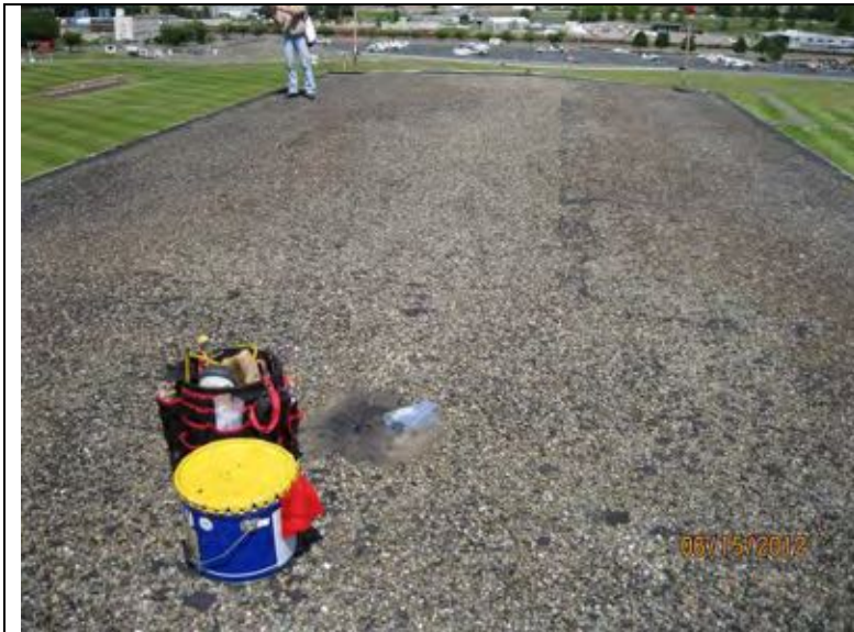
Photograph 8: Upper north roof looking east over the 1918 addition. Test cut in foreground.
