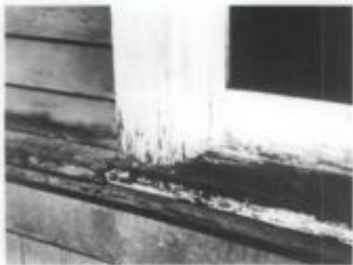
Figure 3. Deterioration of poorly maintained windows usually begins on horizontal surfaces and at joints where water can collect and saturate the wood. The problem areas are clearly indicated by paint failure due to moisture. Photo: Bard M. Smith, AIA
