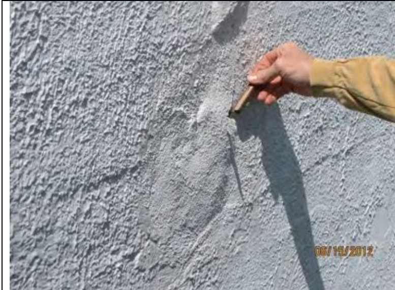
Photo 46: East wall; sealant knife inserted behind delaminated patch material.
