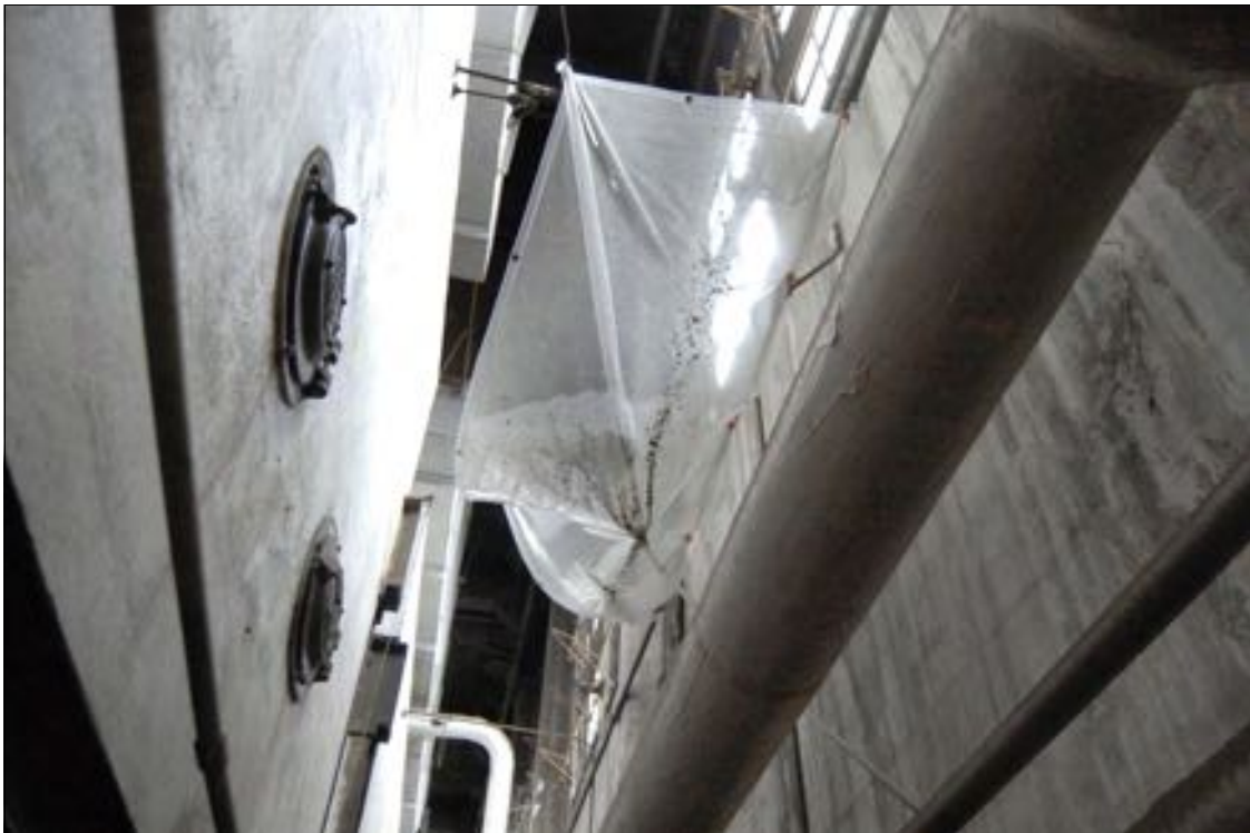
Figure 5. Plastic sheet and pipes used to redirect drain leaks.
