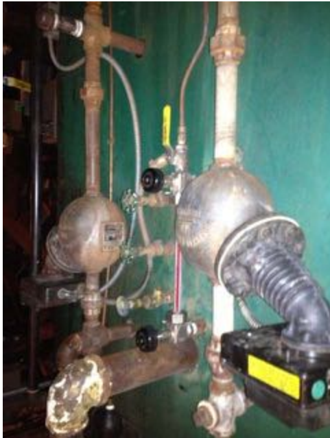
Image 11: Corrosion on boiler, piping
