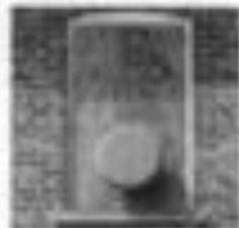
c. The exhaust fan for temperature control.
